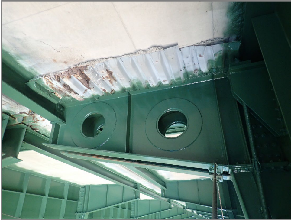
Photo 5 – Base metal at all-around access hole reinforcing plate welds to webs of floorbeam cantilevers (Category E). Floorbeam 26 north cantilever at Girder C shown, looking east.
