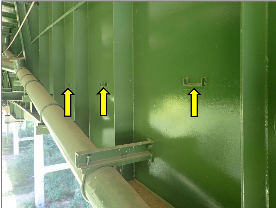
Photo 3 – Base metal at abandoned channel bracket to girder web welds (Category E). Girder C between Floorbeams 52 and 53 shown, looking northwest.
