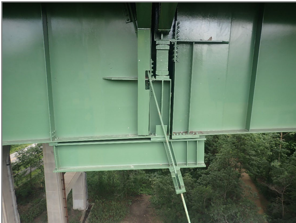
Photo 8 – Typical carrier beam retrofit installed below the seated hinge joints, looking north at Girder A at the Span 4 expansion joint.
