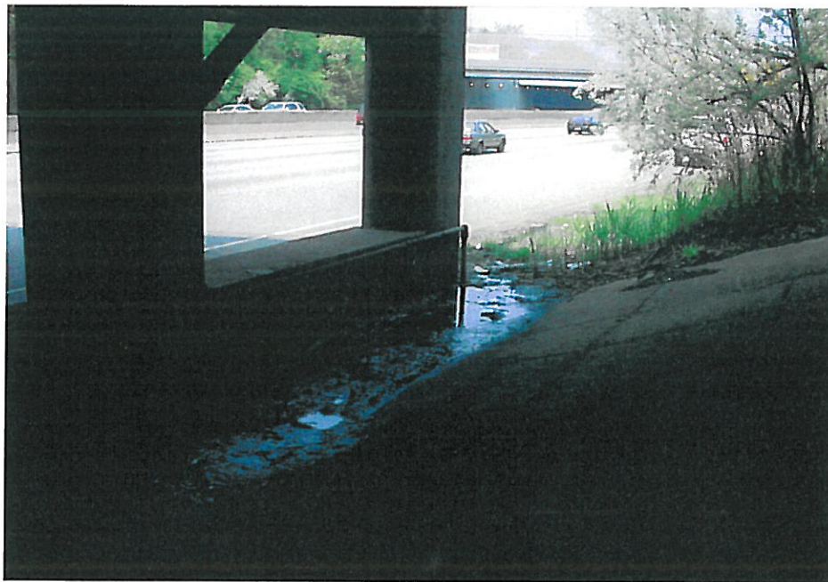
Photo #4 St. Clair Avenue (Eastbound) – Ponded water
