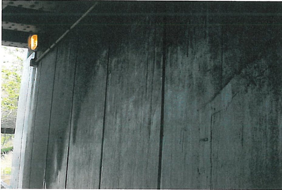
Photo #11 Norfolk Southern Railroad (Eastbound) – Mildew / Cracks
