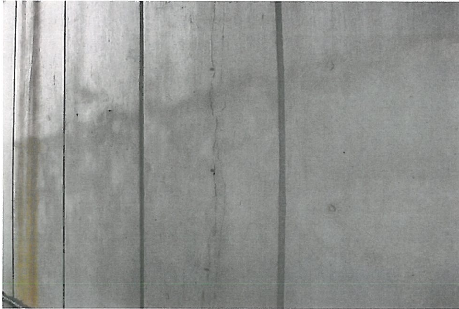
Photo #9 Norfolk Southern Railroad (Westbound) – Cracks and rust stains
