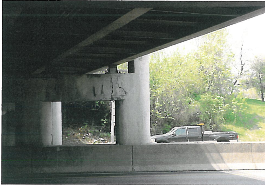
Photo #1 Superior Avenue bridge structure – Distressed pier caps
