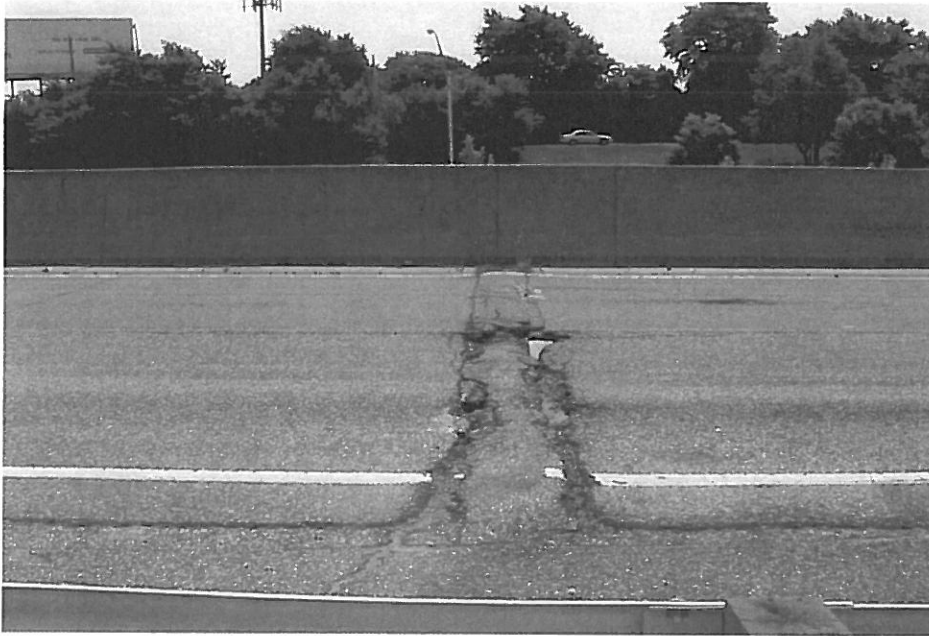
Photo #19 Westbound Memorial Shoreway Interchange (IR-90 overpass) – Distress at approach slab
