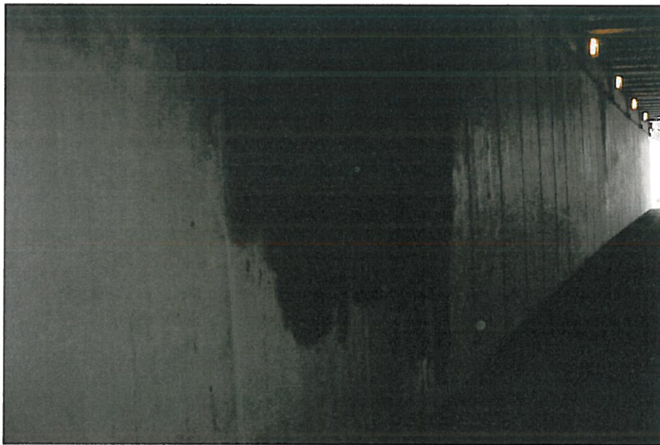
Photo #10 Norfolk Southern Railroad (Eastbound) – Mildew
