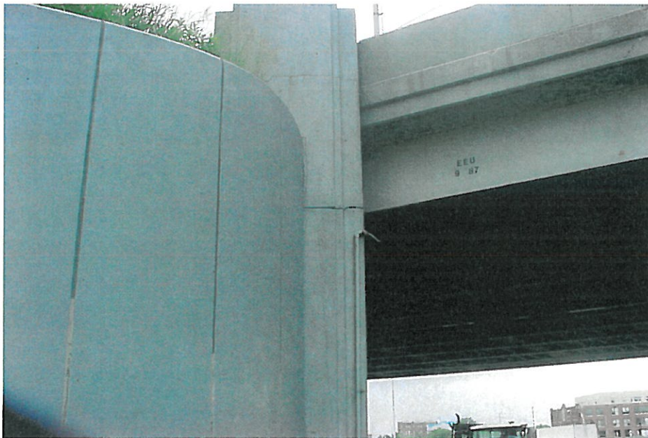
Photo #42 East 55 th Street bridge structure (SE abutment) – Vertical separation below bridge deck
