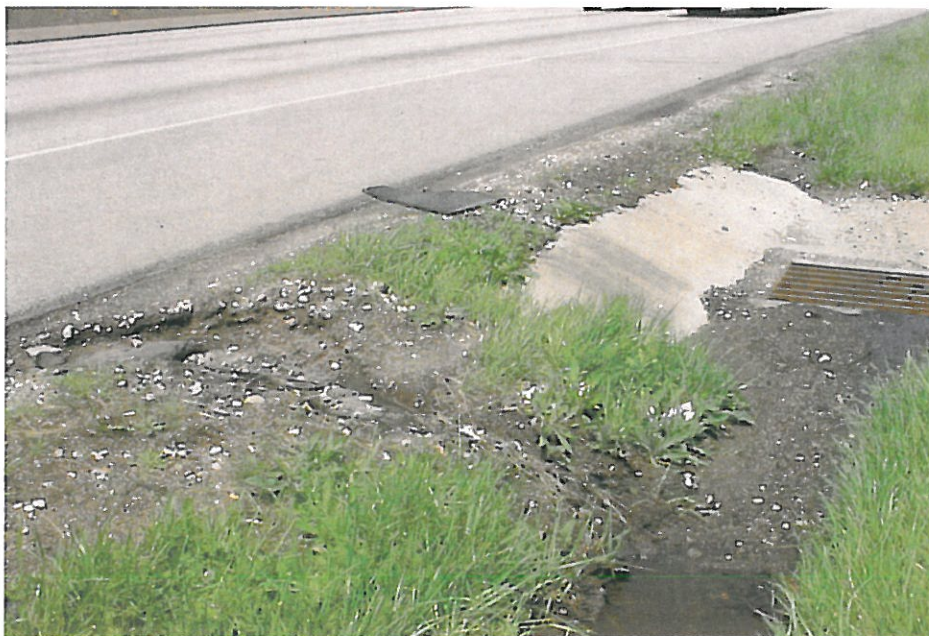
Photo #5 Eastbound IR-90 near Superior Ave. entrance ramp – Roadside erosion
