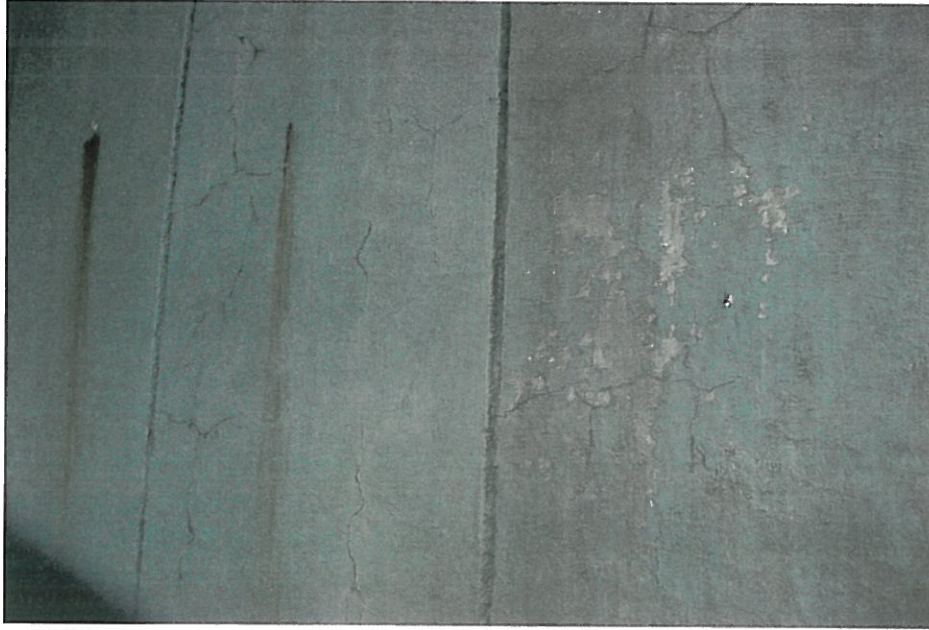
Photo #43 East 55 th Street bridge structure (South abutment) – Cracks and rust stains
