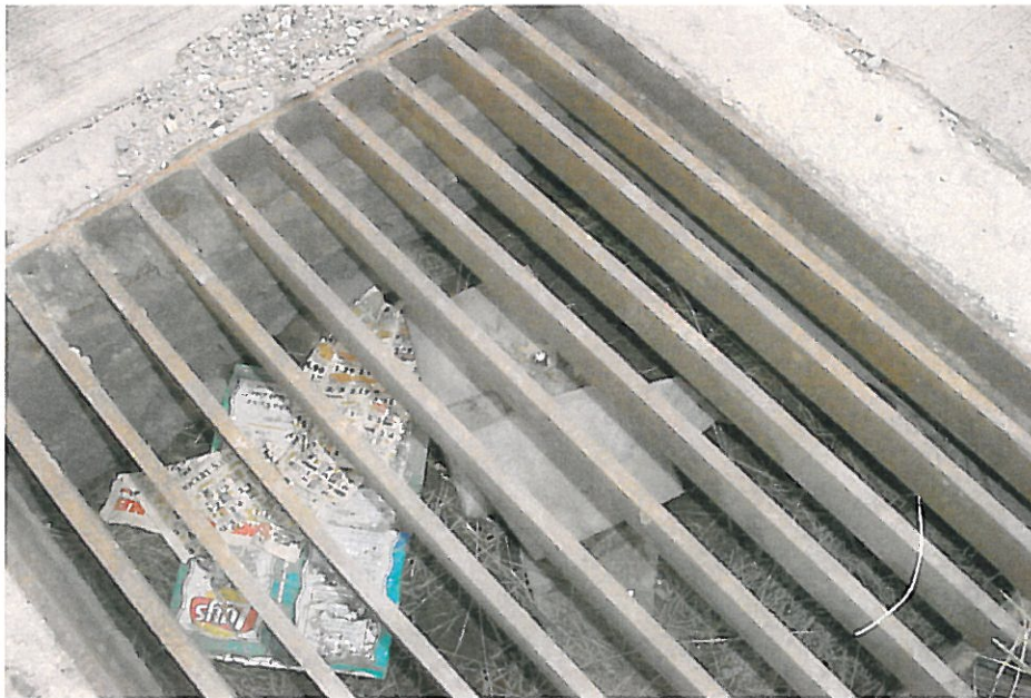
Photo #30 Westbound I-90 (Near Quay 55) – Only top half of outlet and/or inlet pipes exposed
