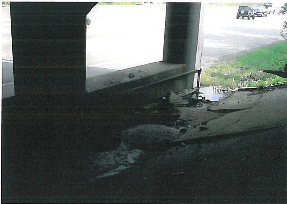
Photo #2 St. Clair Avenue bridge structure (Westbound) – Bridge deck drain outlet below grade
