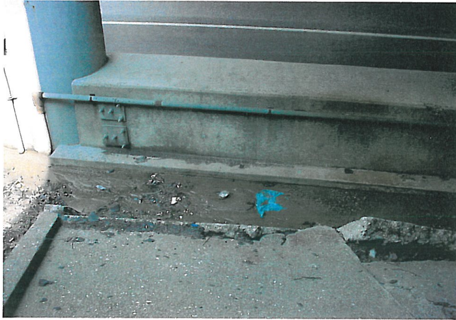
Photo #3 St. Clair Avenue bridge structure (Westbound) - Settled slope protection / Saturated soils
