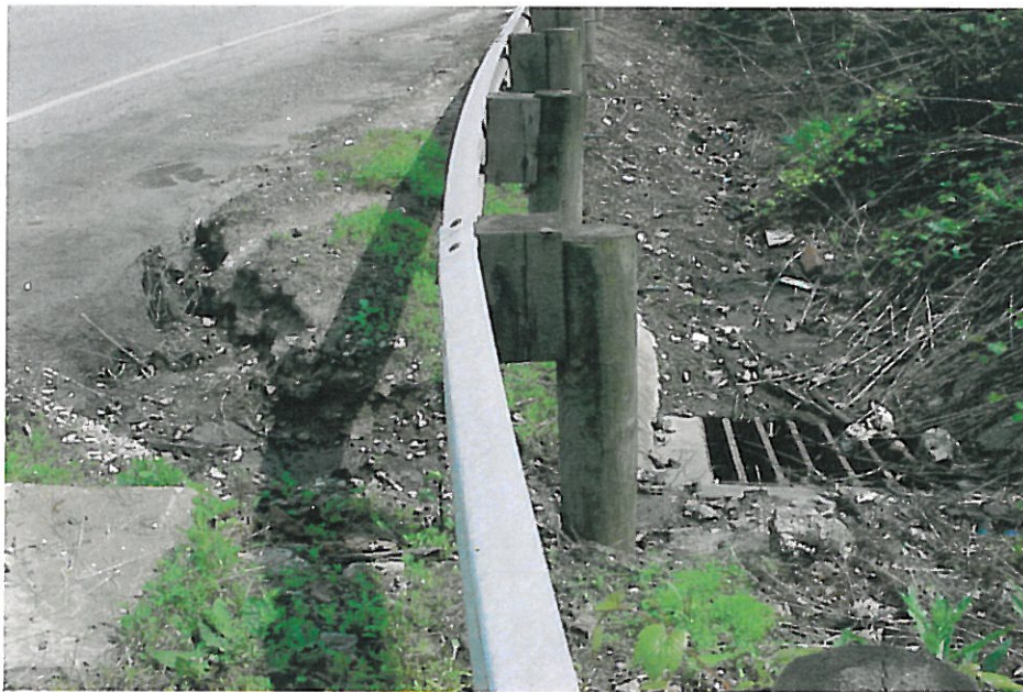
Photo #16 Westbound IR-90 at Lakeside Road entrance ramp – Roadside erosion
