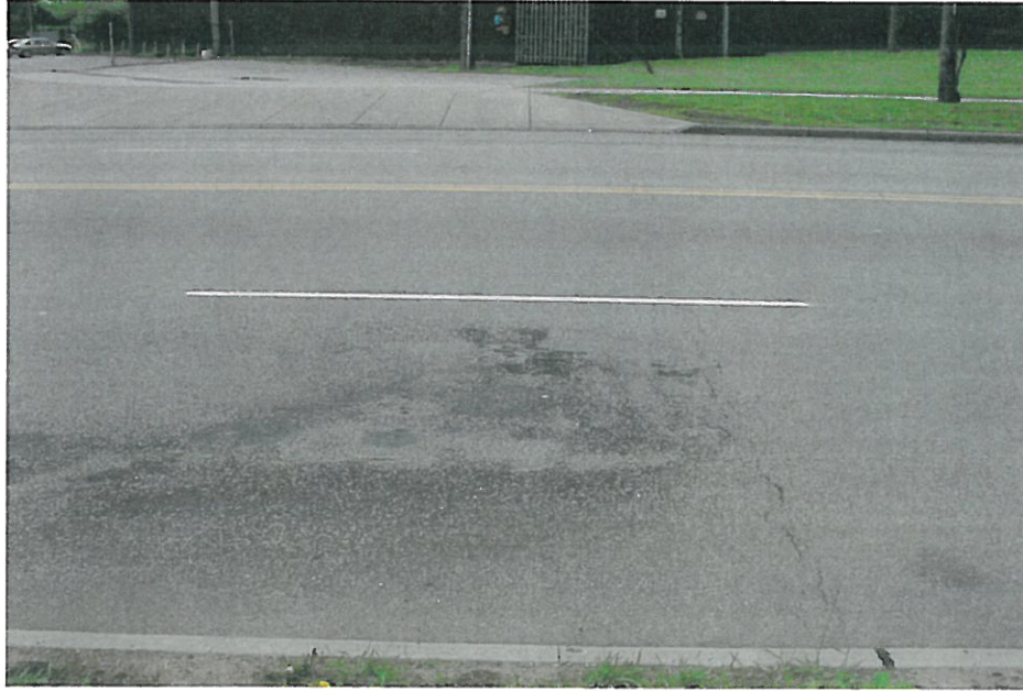
Photo #39 East 55 th Street – Longitudinal crack and surface wear
