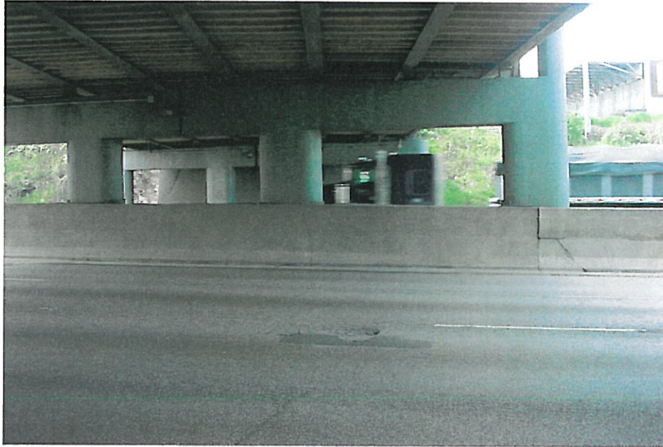
Photo #13 Lakeside Road bridge structure – Cracks in barrier wall below all piers
