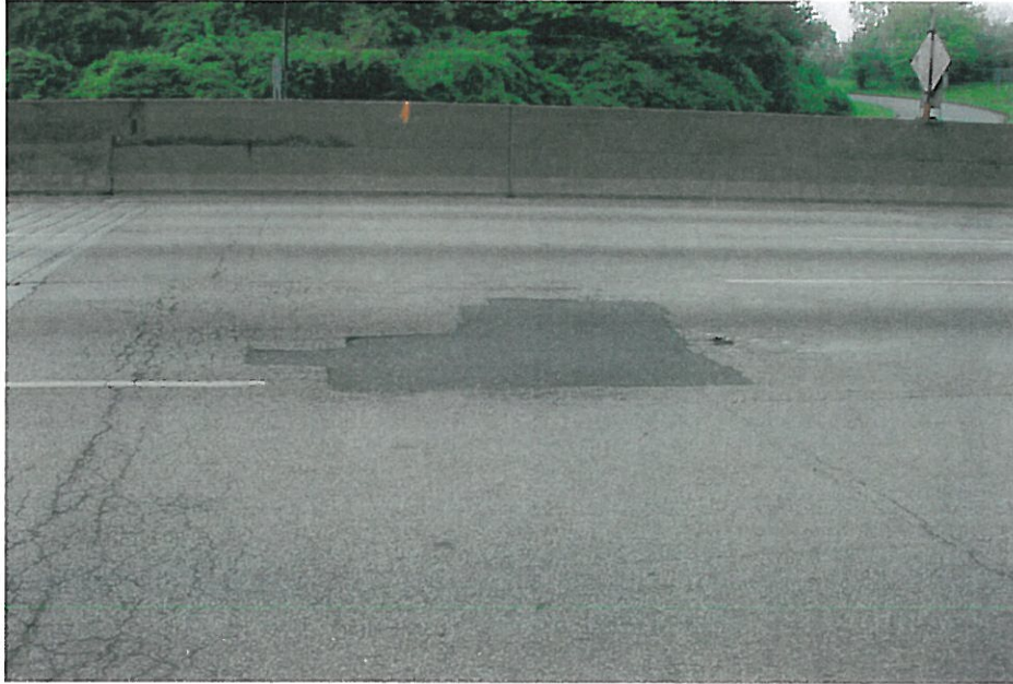
Photo #17 Eastbound IR-90 at Lakeside Road exit ramp – Pavement distress and repair work
