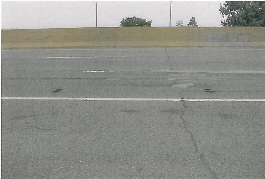
Photo #26 Eastbound Memorial Shoreway (IR-90 west split) – Pavement distress (Typical)
