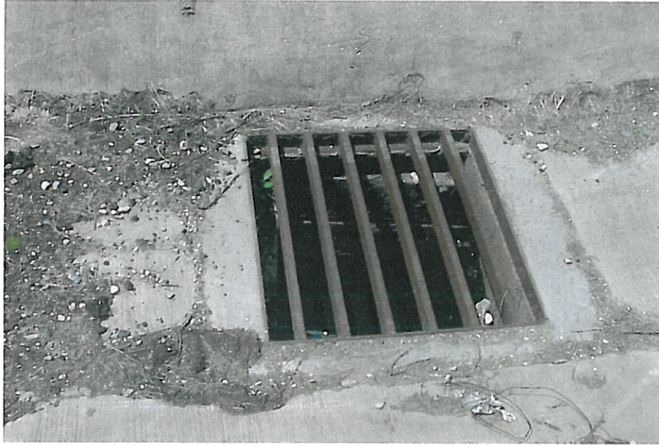
Photo #15 Lakeside Road exit ramp (Eastbound IR-90) – Backed up drain
