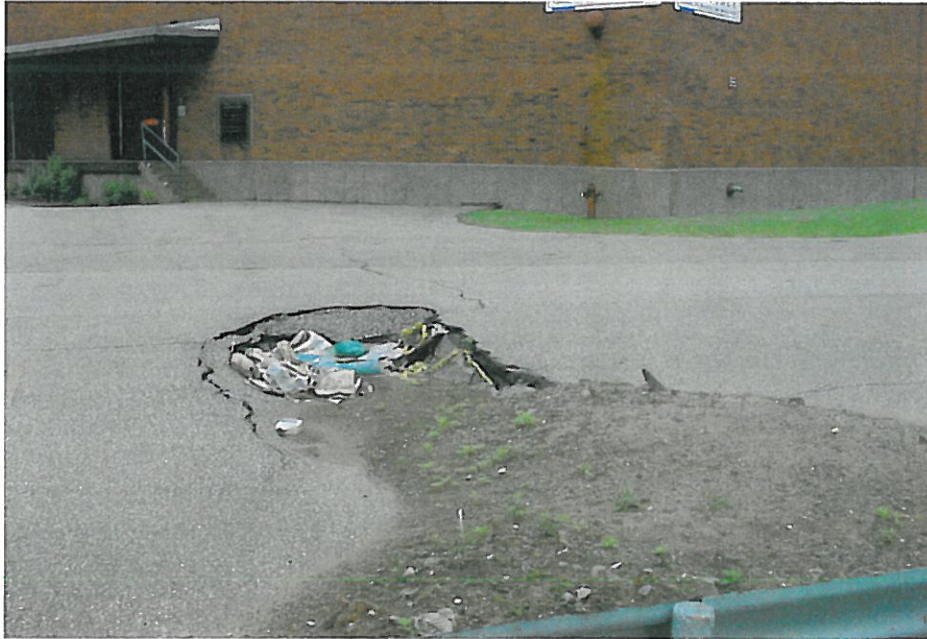
Photo #37 Parking lot immediately north of Lake Court (East 55 th Street) – Sinkhole
