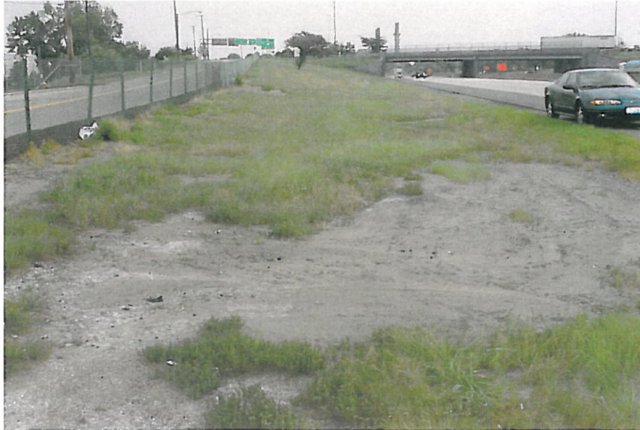
Photo #31 Westbound IR-90 (Adjacent to Photo #30) – Surface erosion
