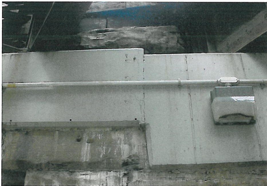
Photo #36 West wall of CSX bridge structure – Hairline crack at joint
