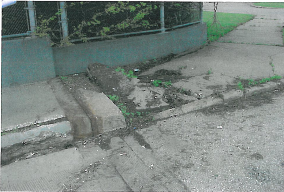
Photo #12 Lakeside Road bridge deck (Northeast section) – Undermined sidewalk
