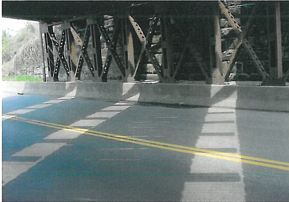
Photo #33 Northbound East 55 th Street under CSX Railroad – Ponded water
