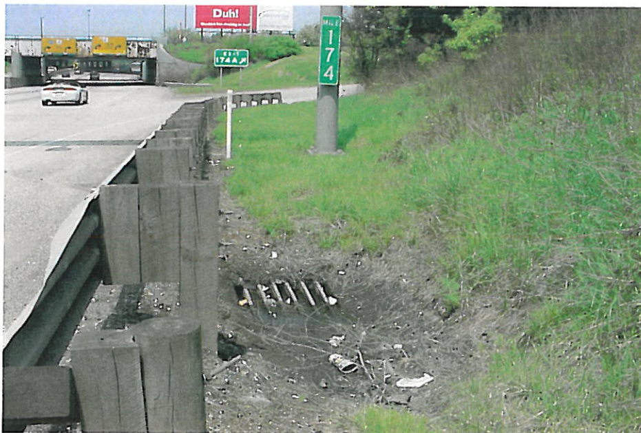
Photo # 14 Eastbound IR-90 approaching Lakeside Road exit ramp – Backed up drain
