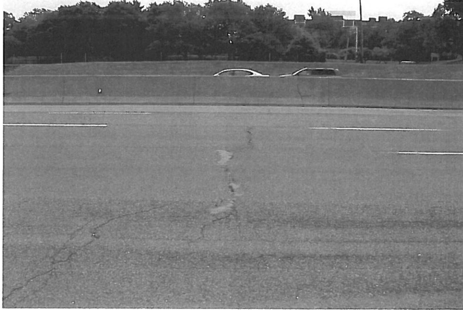
Photo #21 Westbound Memorial Shoreway – Pavement distress (Typical)
