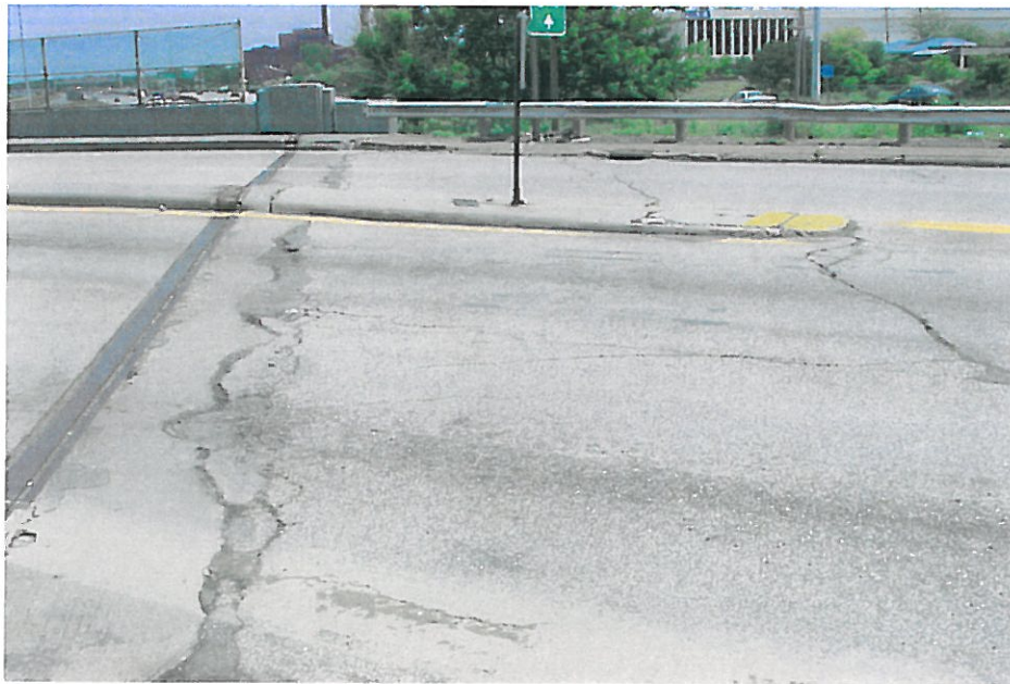
Photo #40 Northbound East 55 th Street approach to IR-90 overpass – Longitudinal cracks
