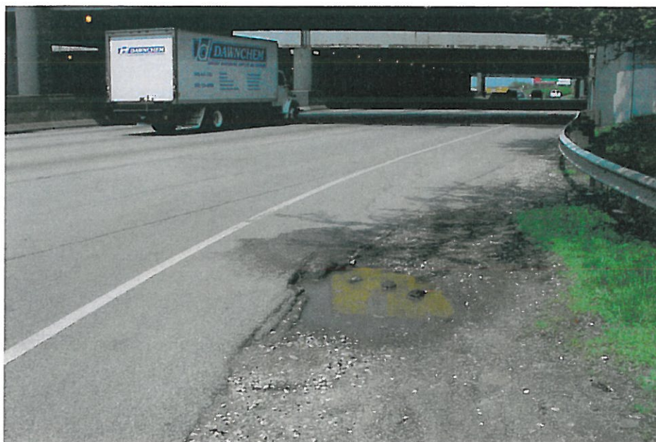
Photo #6 Eastbound IR-90 approaching Hamilton Road overpass – Pothole & ponded water
