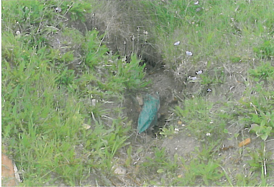
Photo #29 South side of South Marginal Road – Channel erosion and minor slope failure
