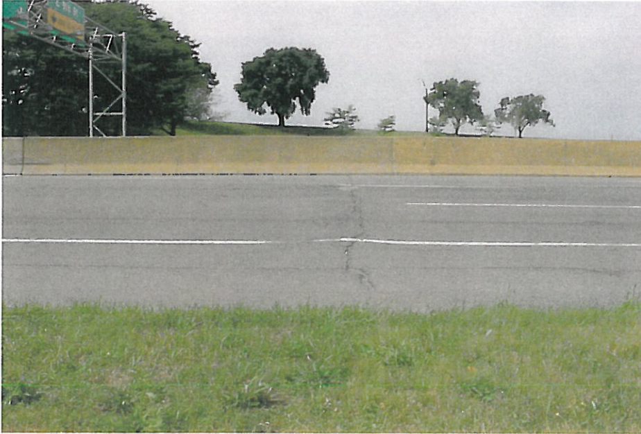
Photo #25 Eastbound Memorial Shoreway – Pavement distress (Typical)
