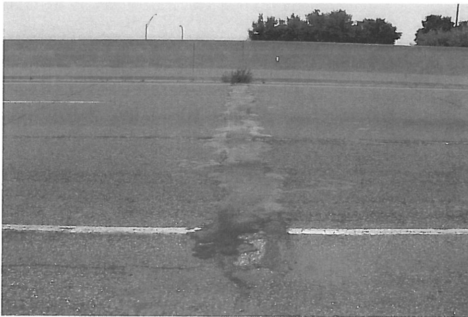
Photo #20 Eastbound Memorial Shoreway Interchange (IR-90 overpass) – Distress at approach slab
