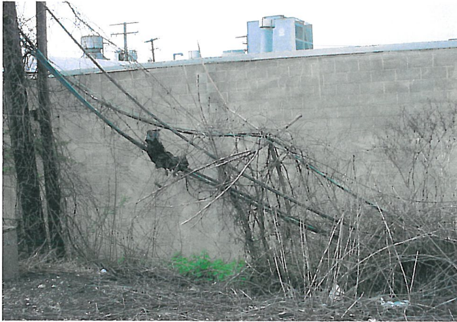
Photo #35 CSX Railroad bridge structure over East 55 th Street – Downed wires
