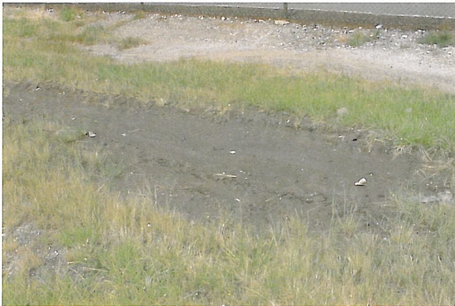
Photo #32 Westbound IR-90 (Adjacent to Photo #31) – Wet area
