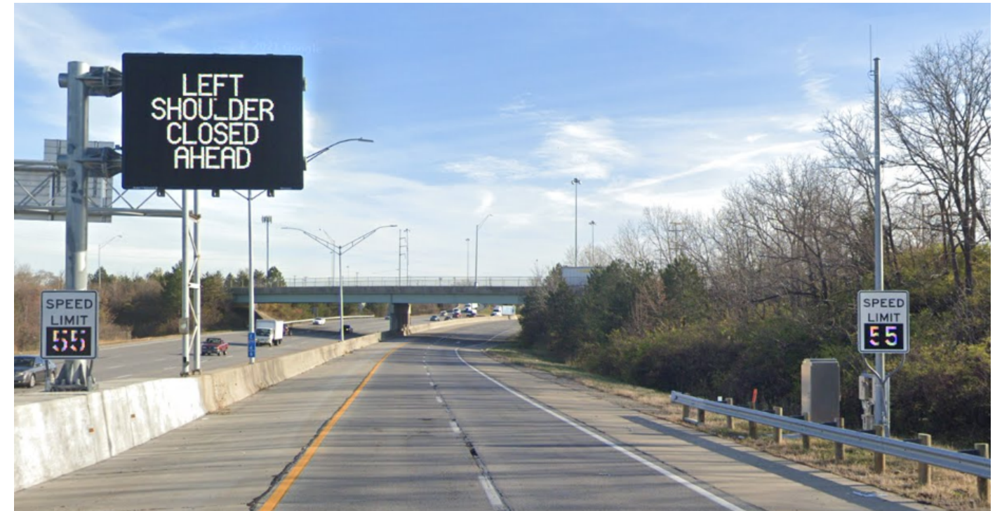
Figure 15 – Cantilevered DMS board used on I-670 SmartLane
