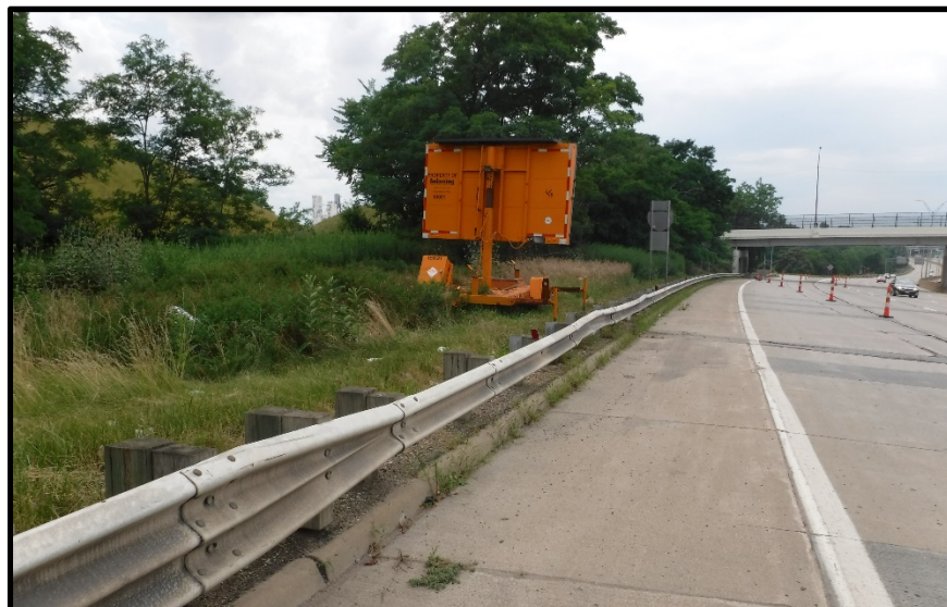
Photo 5 – Eastbound Mainline West Abutment, South shoulder guardrail damage
