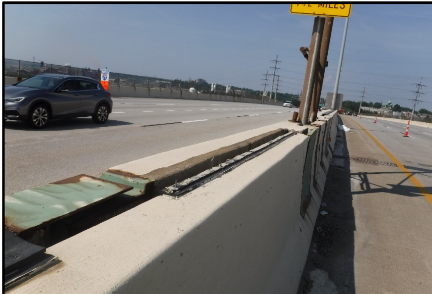
Photo 13 – Neoprene cover missing from the top of the median
