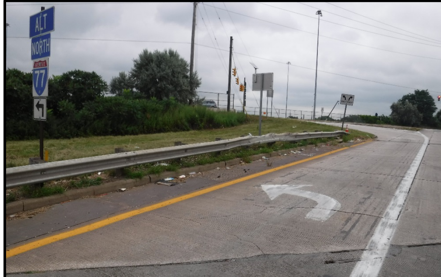
Photo 4 – Collision damage at the North side of the Eastbound Ramp C-B guardrail
