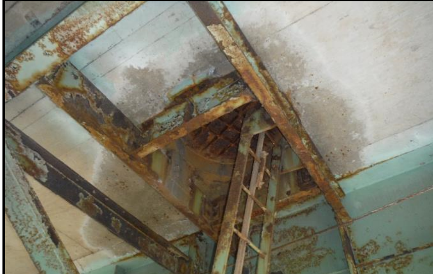
Photo 9 – Manhole at Pier 14R with saturated concrete and minor rust staining
