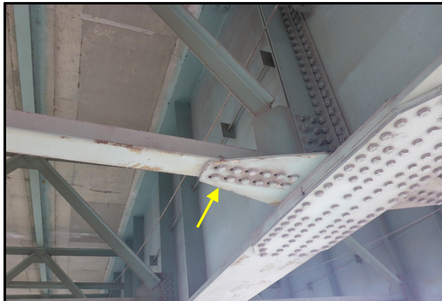
Photo 42 – Floorbeam misdrilled holes at connection plate
