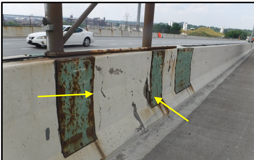
Photo 14 – Spalled and cracked median with exposed reinforcing steel at sign support plates
