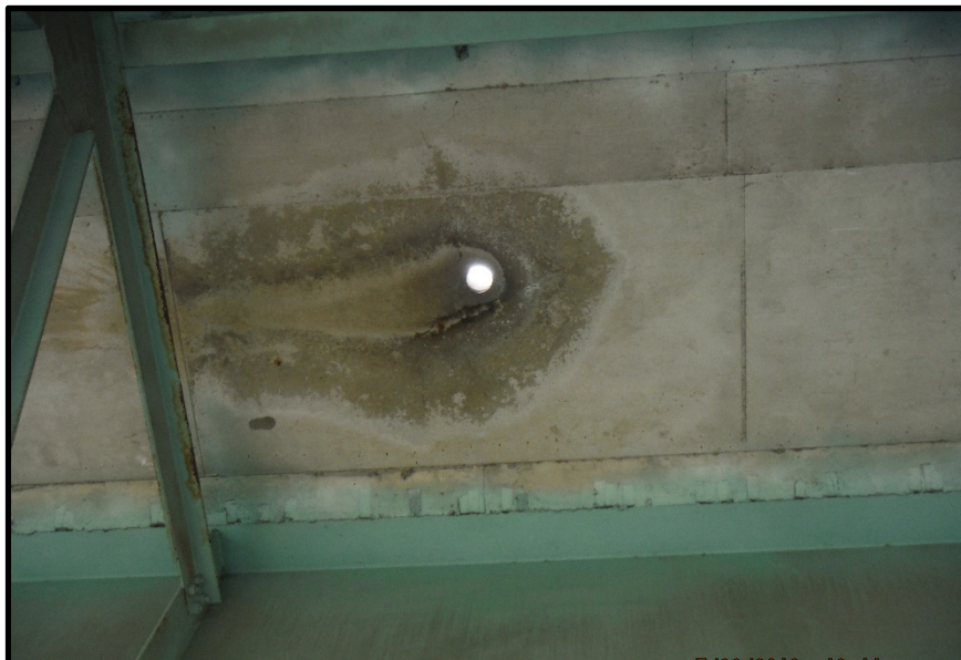
Photo 10 – Open deck core with saturated concrete West of Pier 10
