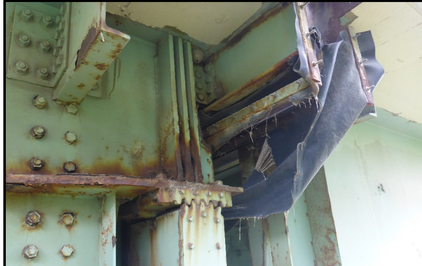
Photo 21 – Torn neoprene sheeting causing debris to spill onto the steel below
