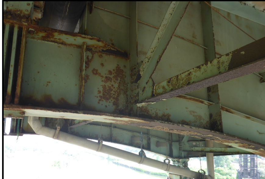
Photo 36 - Crossframe corrosion near Expansion Joint
