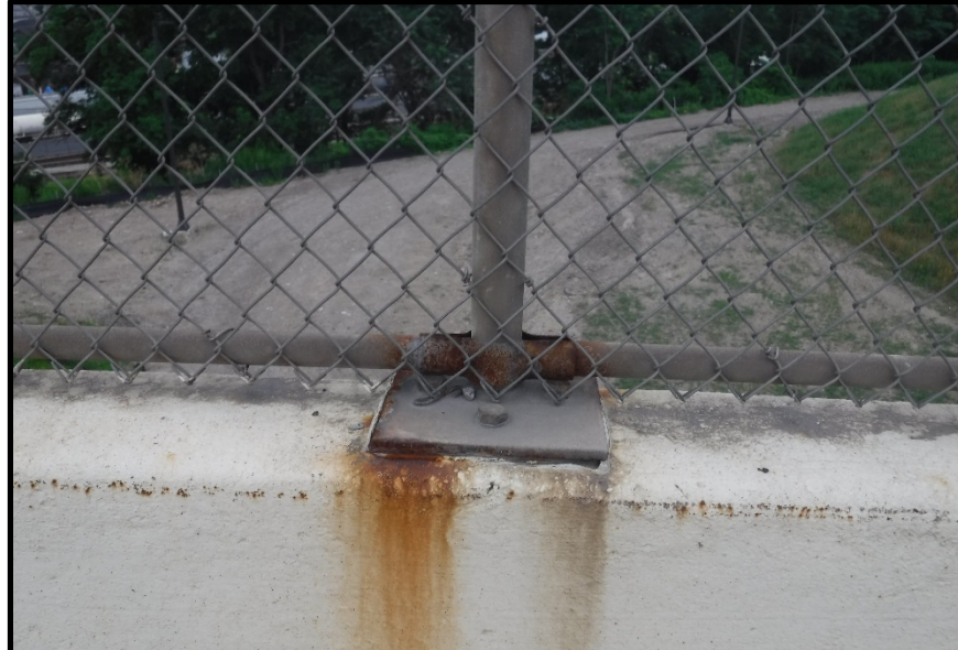
Photo 17 – Fence base plate separating from concrete in Span 5
