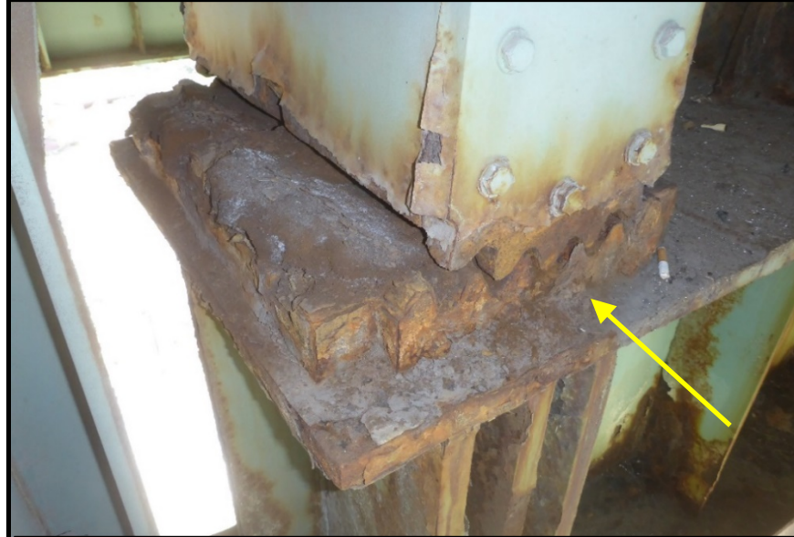
Photo 54 – Expansion Hinge 3 Girder D missing or broken bolts
