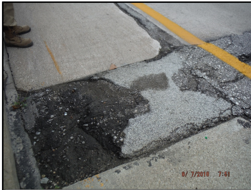
Photo 3 – The Westbound mainline forward relief joint which is deteriorating in the shoulder
