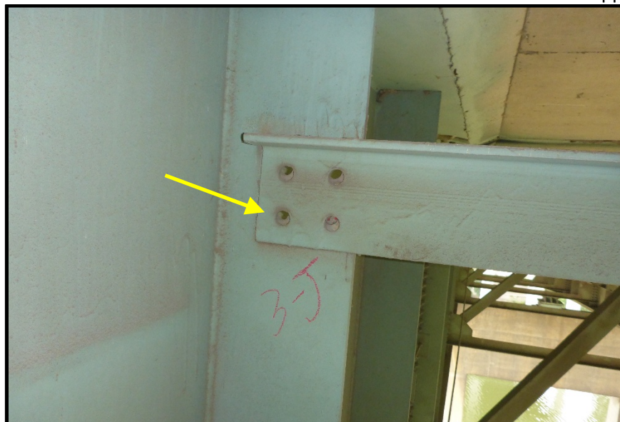
Photo 37 - Crossframe missing bolts in Unit 3 Span 3
