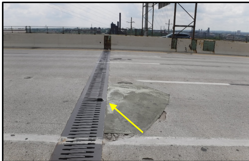
Photo 26 – Missing teeth at Westbound Expansion Joint 2; also note deck patch.
