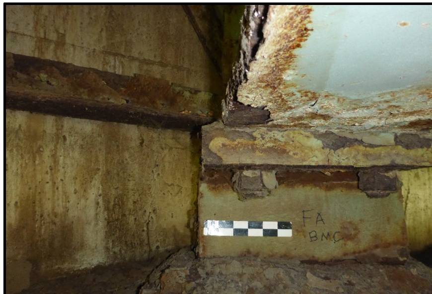
Photo 47 – Forward Abutment Bearing Off Center
