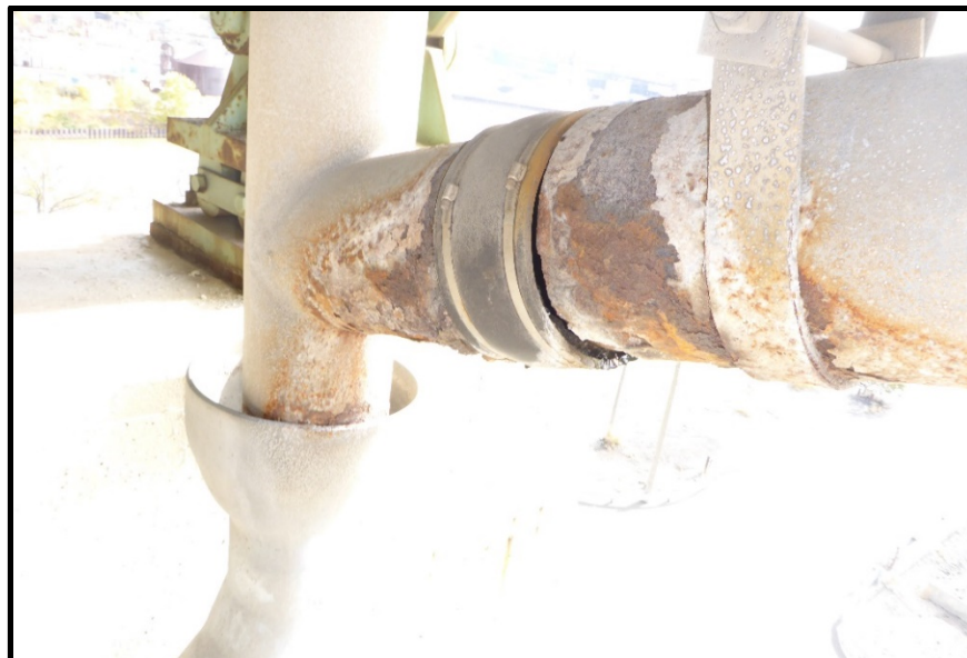
Photo 22 – Misaligned coupler at Pier 9 drainage spout
