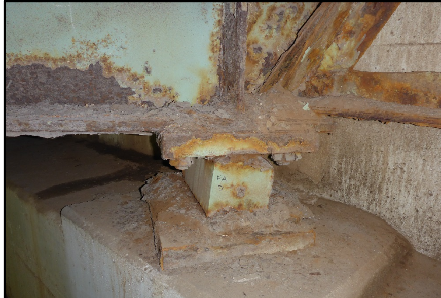
Photo 46 – Laminar corrosion on base plate and bolts of bearings
