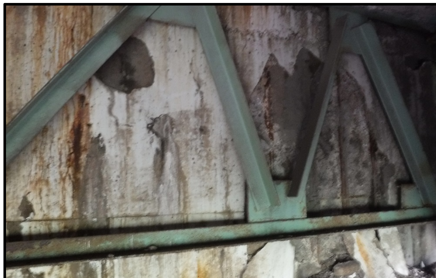
Photo 28 – Deterioration to Forward Abutment Backwall below sliding plate joint
