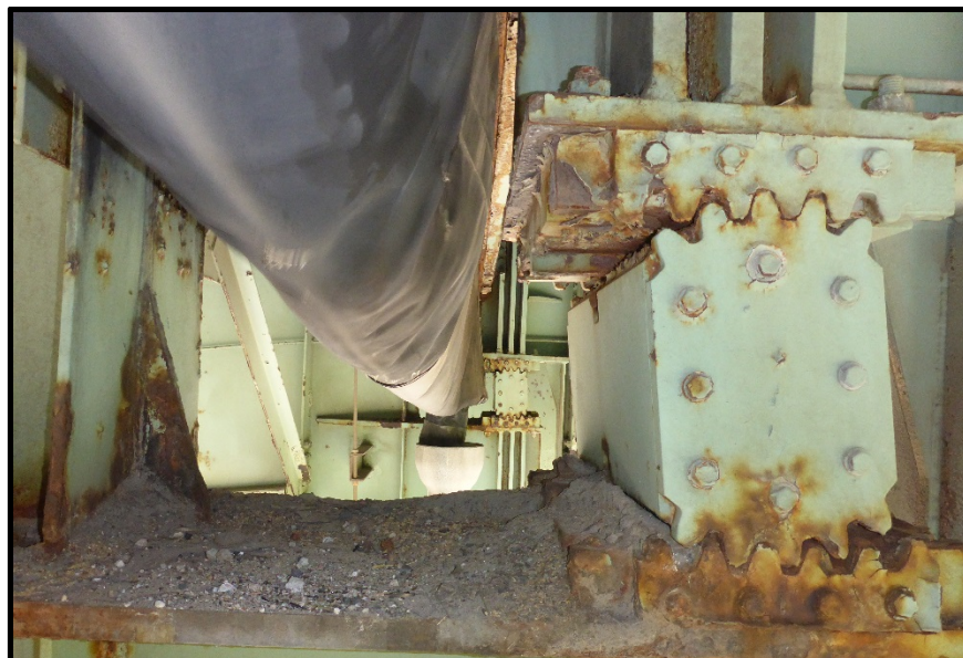
Photo 55 – Debris Piled on Girder Flange around hinges
