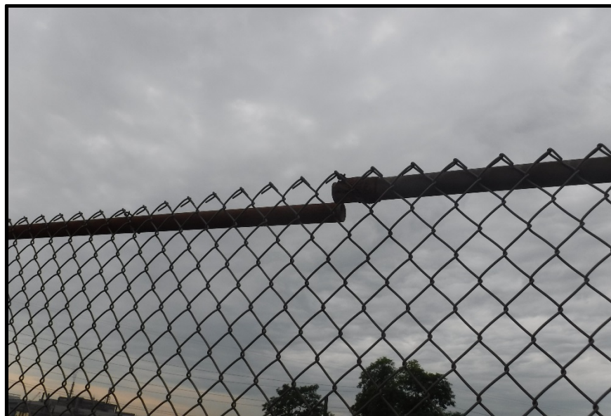
Photo 18 – Bottom railing failed due to corrosion at Span 14
