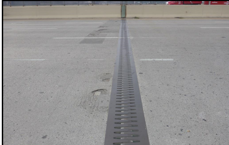
Photo 25 – Transversely misaligned steel teeth at Westbound Expansion Joint 5
