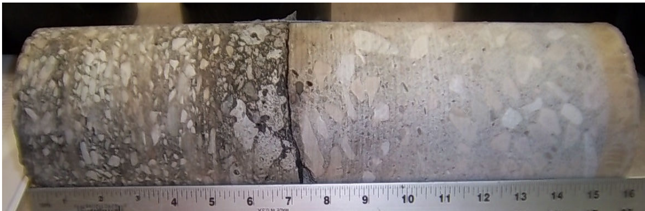
Core #35 Location: NW, Center on Professor Ave. 7 ¼" Asphalt / 8 ¾" Concrete
