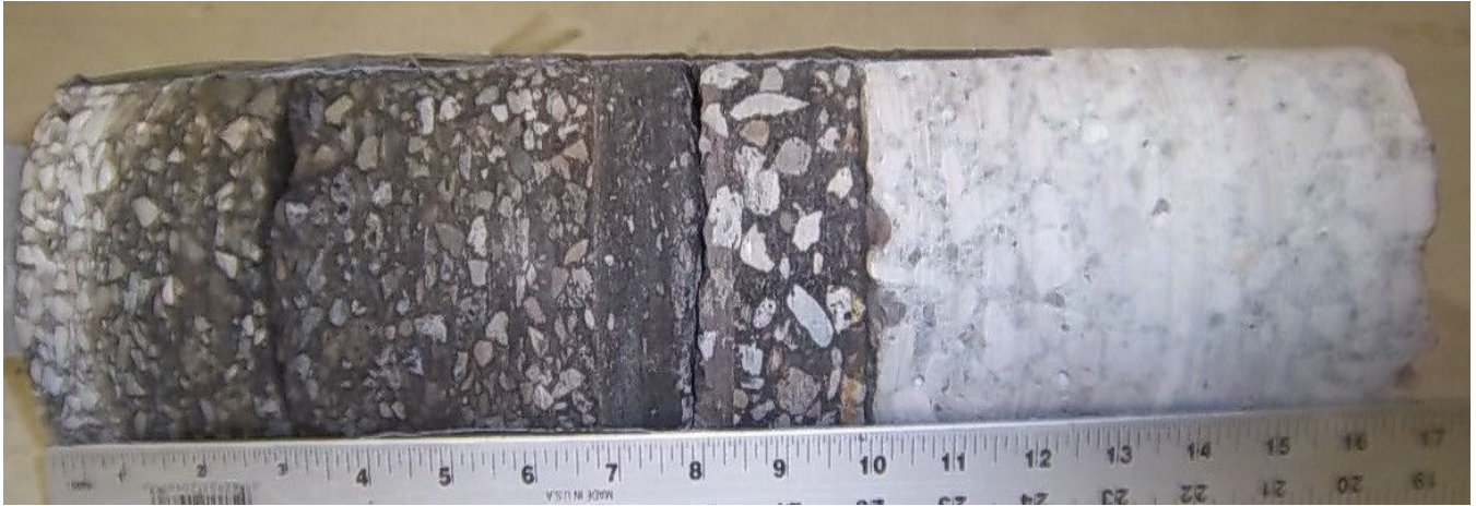
Core #64 Location: Center of W. 6 th St. and W. St. Clair Ave. 10" Asphalt / 6 ½" Concrete
