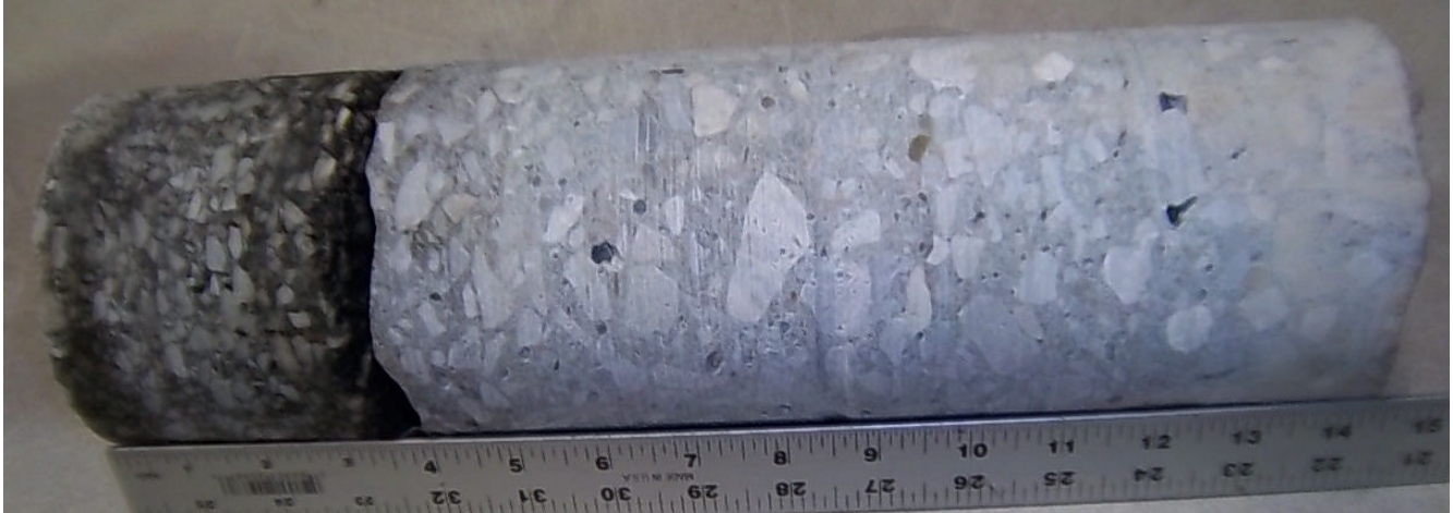
Core #65 Location: East Side of W. 6 th St. and W. St. Clair Ave. 3 ½" Asphalt / 11" Concrete
