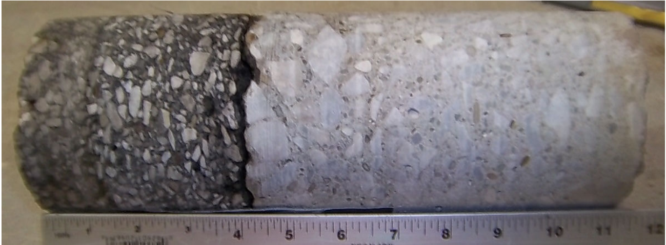
Core #54 Location: West Side of W. Lakeside Ave. and W. 6 th St. 4 ¼" Asphalt / 7" Concrete
