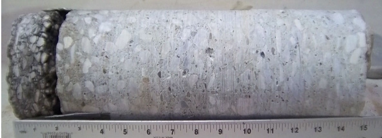
Core #57 Location: West Side of W. 6 th between W. Lakeside Ave. and Johnson Ct. 2" Asphalt / 13" Concrete
