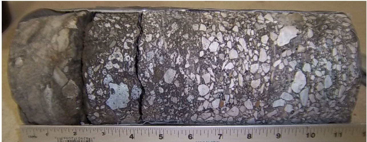
Core #56 Location: East Side of W. Lakeside Ave. and W. 6 th St. 11 ¼" Asphalt
