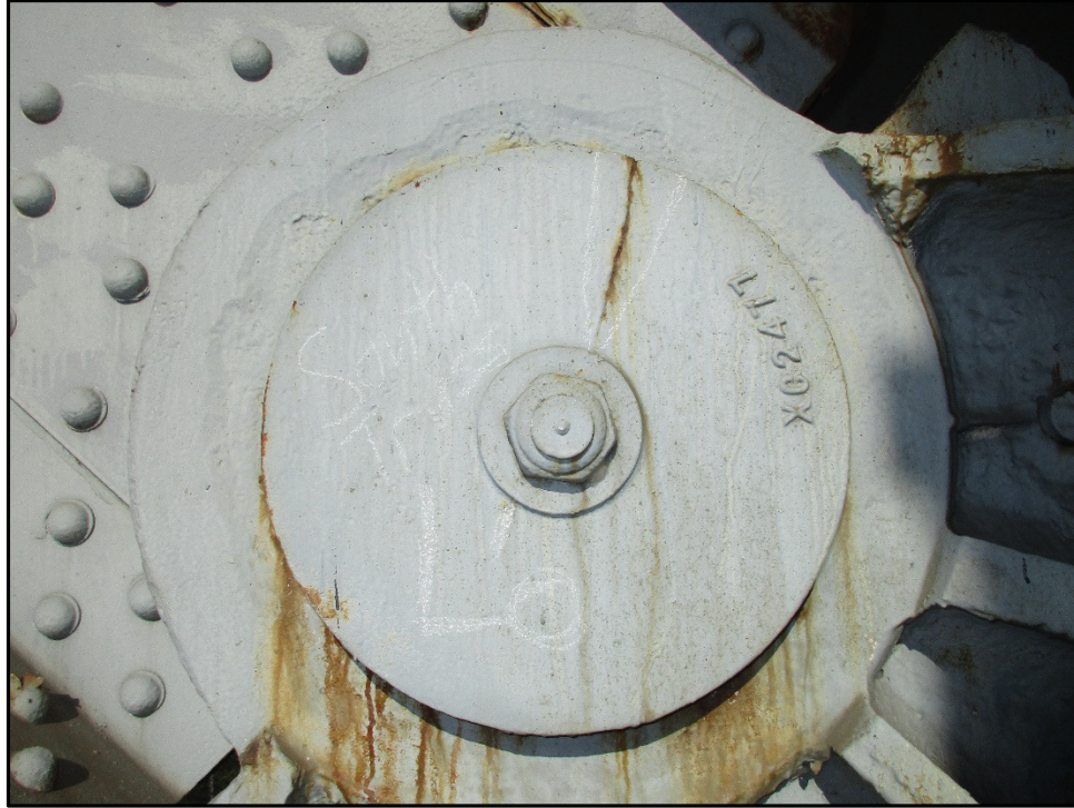
Photo 42 – Typical Bearing Pin Cover Plate Crack.
