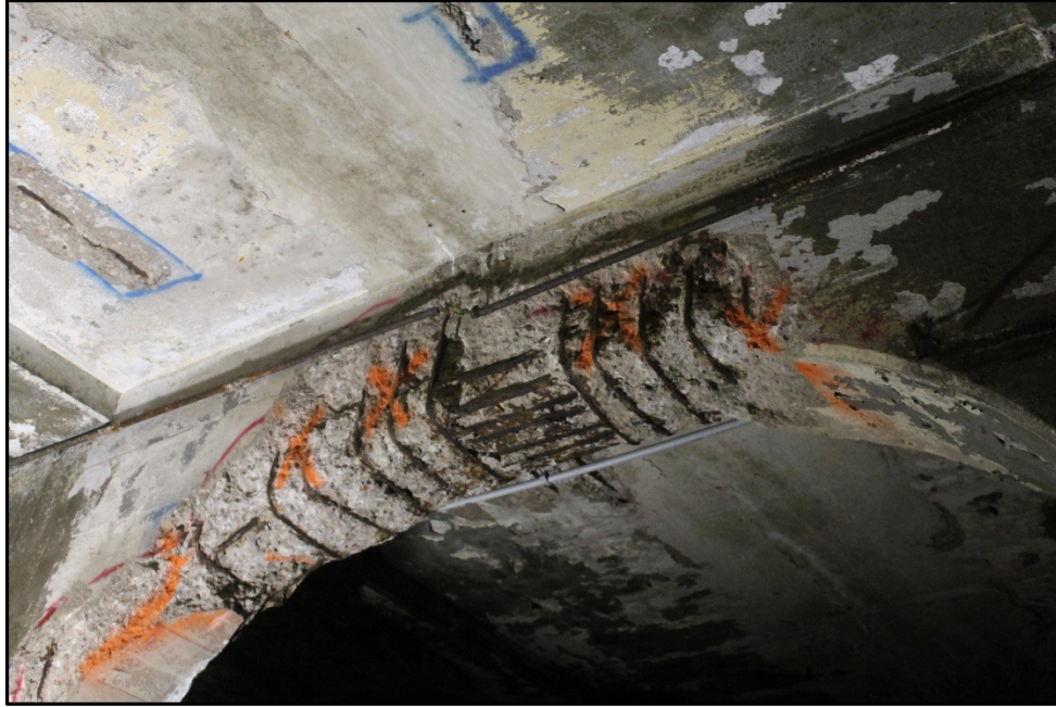
Photo 31 – Spalled Beam D22, West Station.
