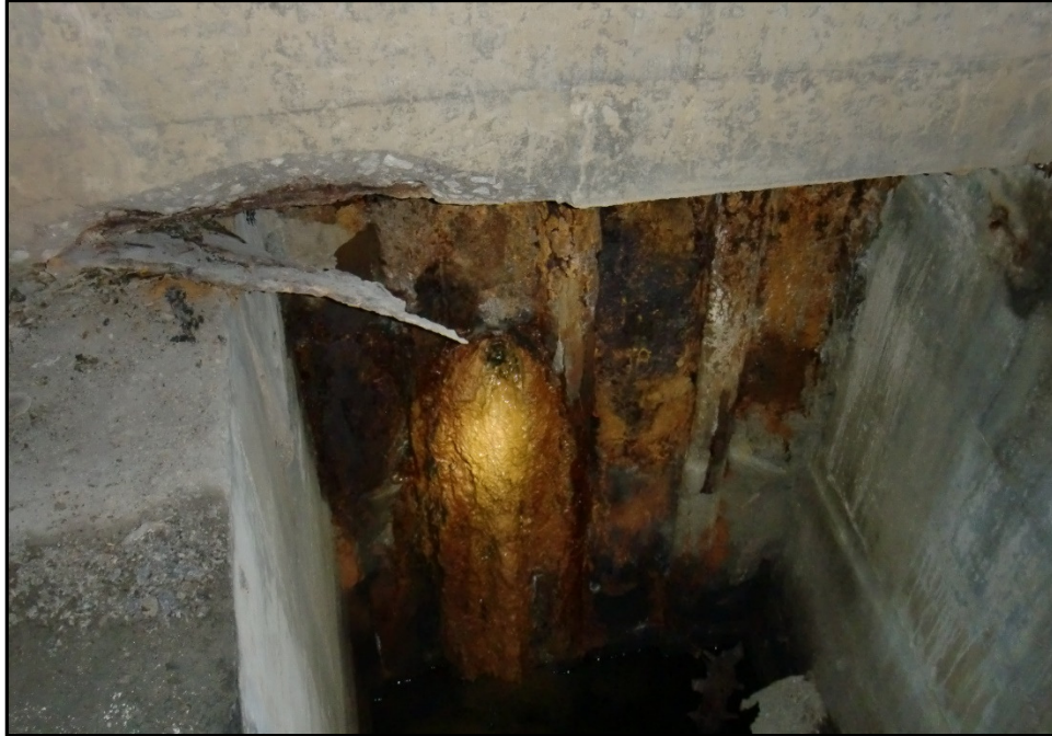
Photo 45 – Possible Deposit Clogged Pedestrian Tunnel Drain Outlet, East Abutment Cellular Construction.
