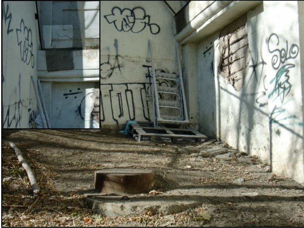
Photo 55 – Improvised Access Ladder on East Face, Tower A South.
