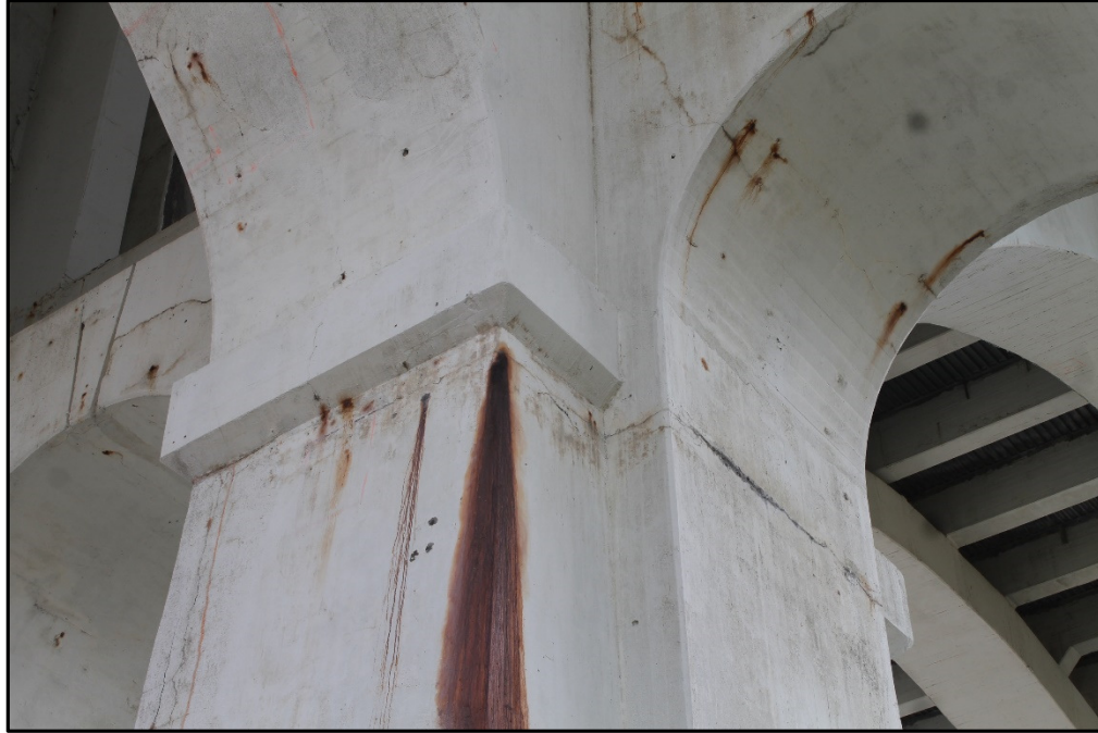
Photo 50 – Rust Stains Indicating Active Corrosion of Pier Reinforcement.
