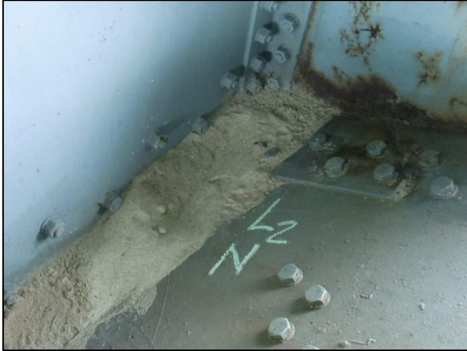
Photo 44 – Blast Material Accumulation, Top of Lower Lateral Bracing Gusset Plate, Panel Point North L2.
