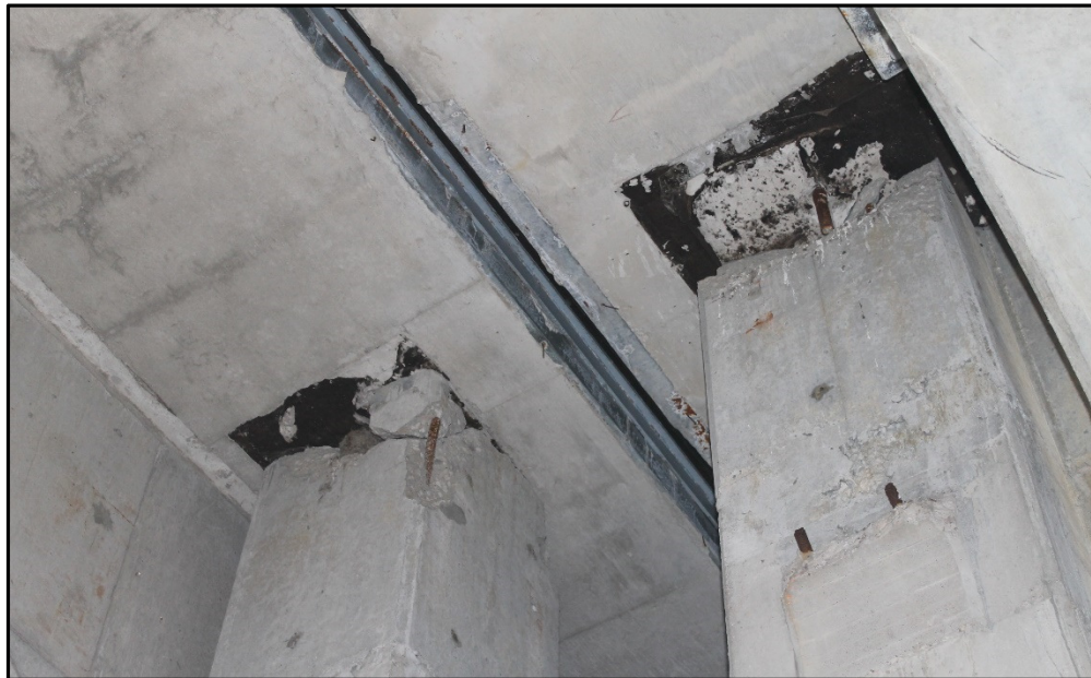
Photo 53 – Fracture of Top Interior Section Against Upper Deck Slab, Tower B South.
