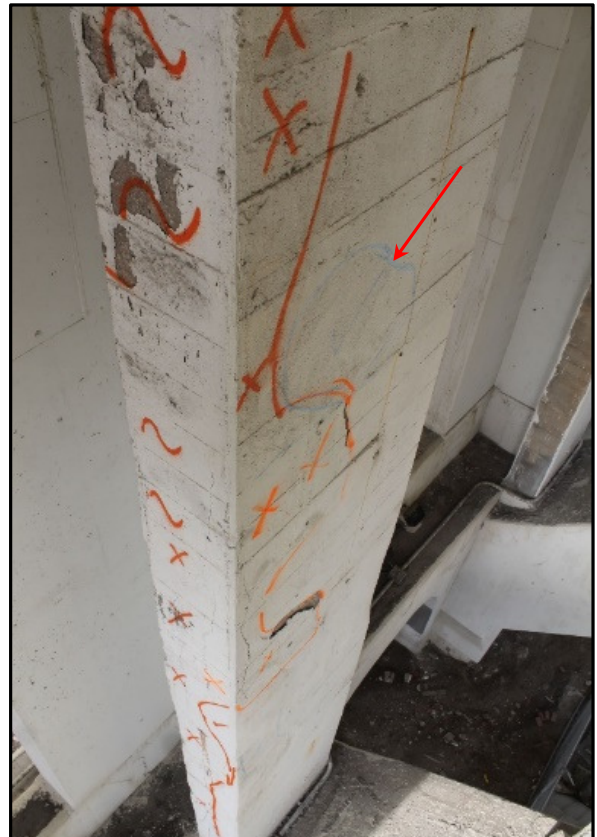
Photo 26 – Delaminated Surfaces Surrounding 1995 Patch Area (at Arrow), Lower Deck Column SE 1, Span 3.
