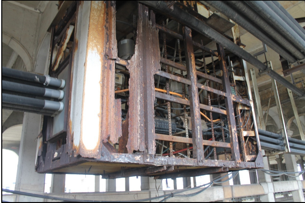
Photo 59 – Corroded & Unsecure Telephone Junction Chamber, Span 2 Lower Deck.
