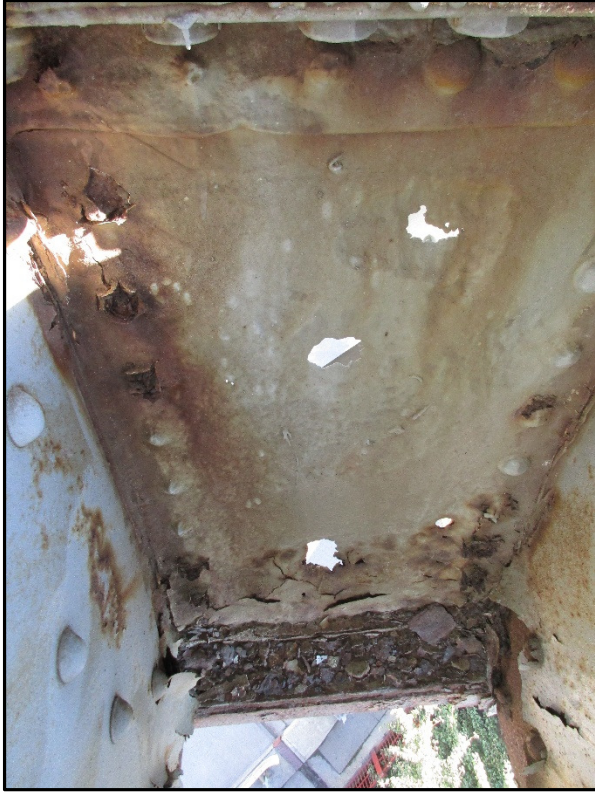
Photo 34 – Common Perforations of Lower Chord Diaphragm.
