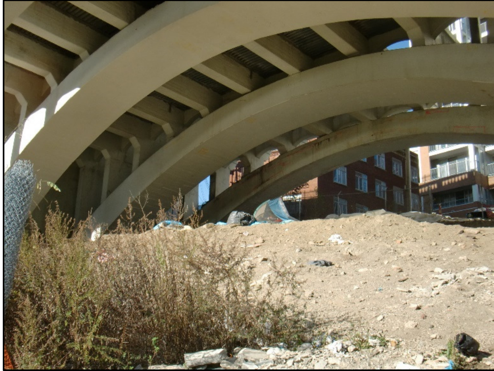
Photo 58 – Homeless Tents Within Intended Span 1 Secure Zone.
