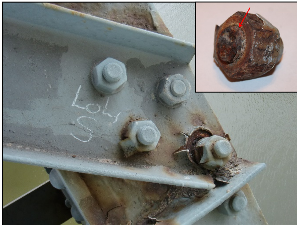
Photo 37 – Fractured Bolt, South LoL1. (Inset: Fracture Origin at Arrow.)
