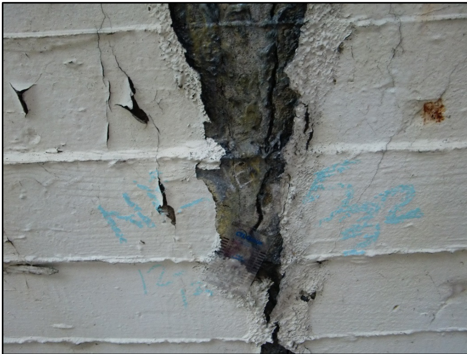
Photo 21 – Close-up of \frac{5}{32} " Open Epoxy-Injected Intrados Crack, Panel 13, NE Arch Rib, Span 5.
