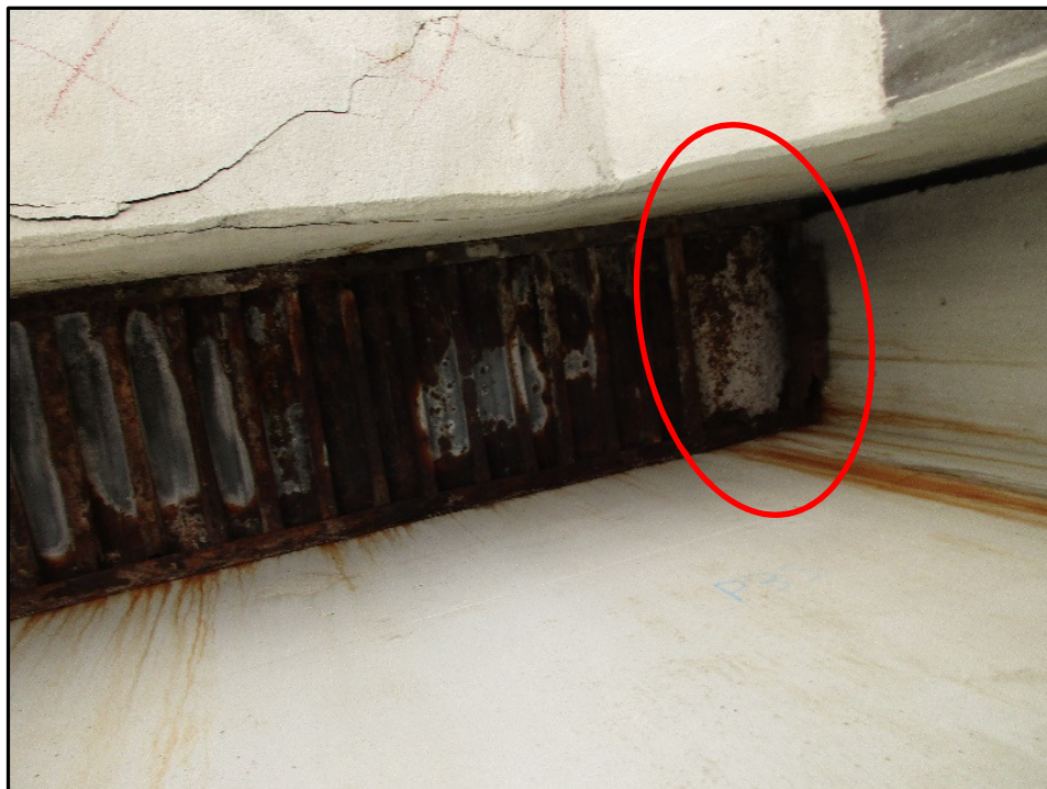
Photo 9 - Corroded & Missing Stay-in-Place Form (Circled), Lower Deck Panel 15 Center, Span 2.
