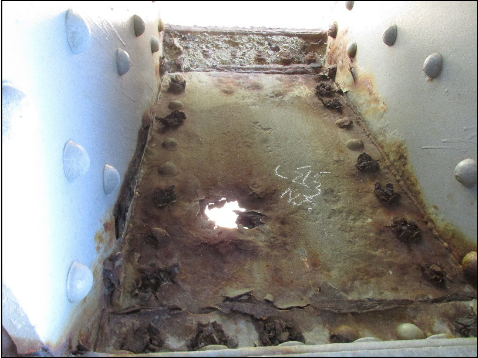
Photo 35 – Common Perforations of Lower Chord Diaphragm & Debris on Lower Transverse Angle.
