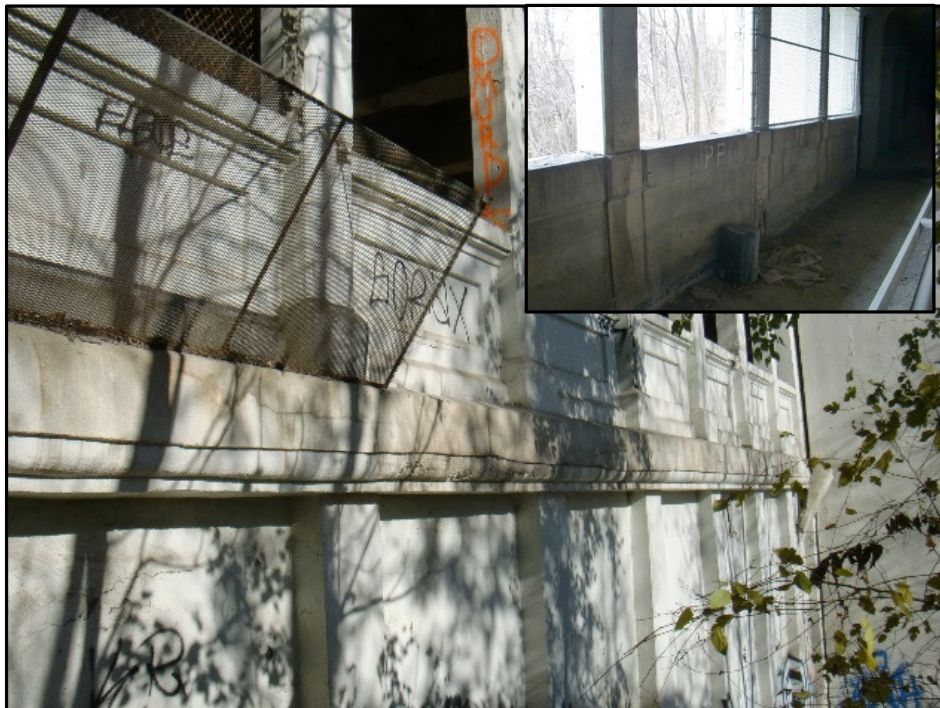
Photo 56 – Continuation of Unauthorized Access to Span 1A Lower Deck.
