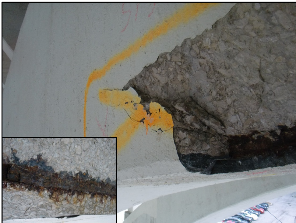
Photo 23 – Sound 1996 Shotcrete Patch & Fractured Original Concrete, SI Arch Rib, Span 7.
