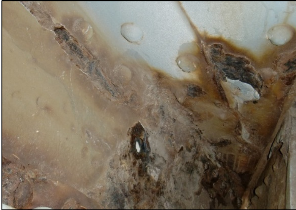
Photo 39 – Typical Rust Nodule (at Arrow) on Interior Gusset Plate Surface.
