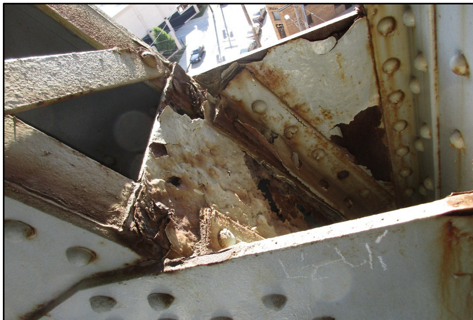
Photo 33 – Minor Pitting Top Stay Plate, U1'-L2' South.
