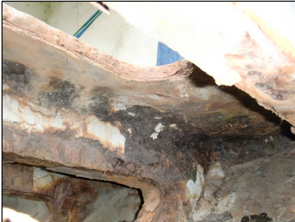
Photo 43 – Typical Corrosion Interior Surface of Bearing Casting.
