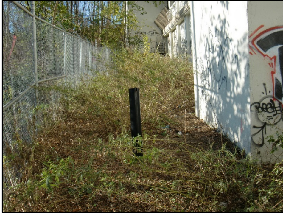
Photo 3– Slope Inclinometer, Tower B South.
