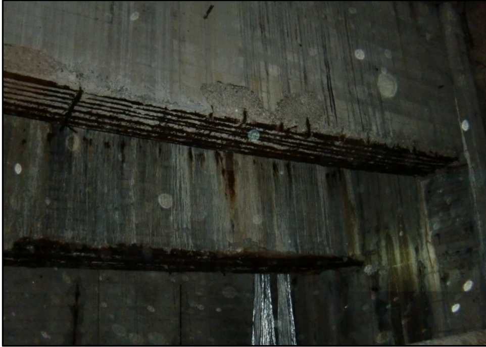
Photo 30 – Exposed Bottom Reinforcement Mat, Lower Deck Floorbeams 1 & 2, East Station.
