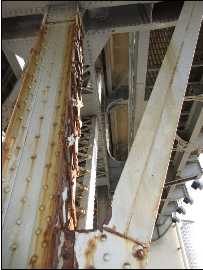
Photo 32 – Typical Minor Corrosion of Vertical Below Lower Deck.
