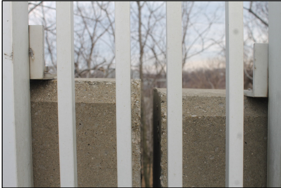
Photo 15 – Uneven Top of South Rail, Tower A.
