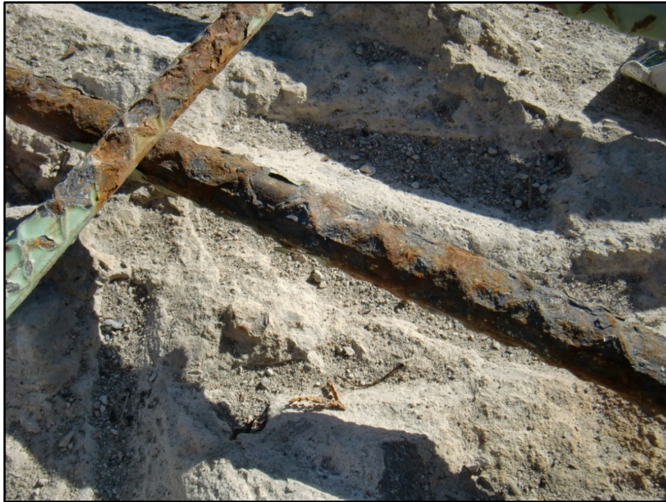
Photo 7 – 1/8-inch Section Loss of Epoxy Coated Rebar Following 18 years of Service.
