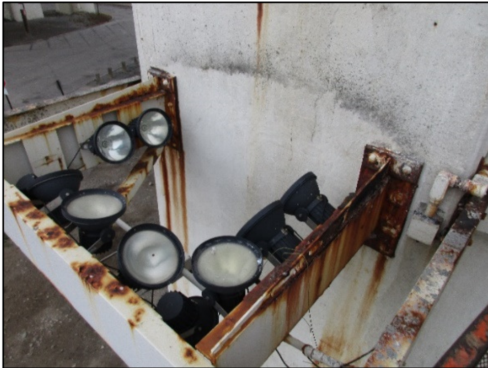
Photo 60 – Typical Paint Failure & Corrosion, Exterior Pier Shaft Lighting Brackets.
