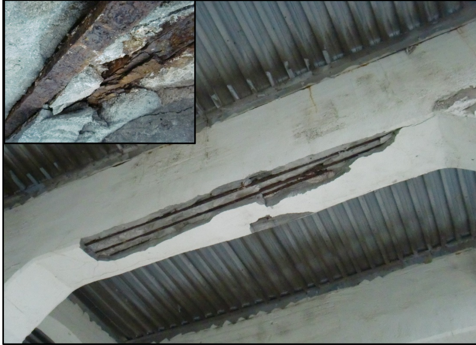
Photo 28 – Spalled 1996 Shotcrete Patch, Lower Deck Floor Beam 14, South Bay, Span 6. (Inset: Continued reinforcement corrosion at shotcrete patch-original concrete interface.)
