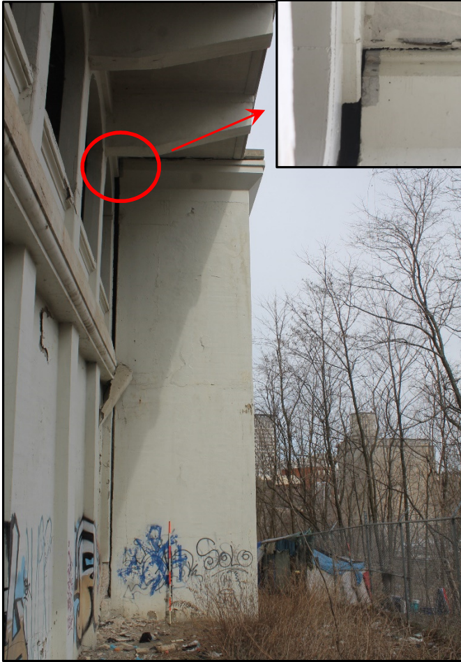
Photo 52 – Rotation of Tower B South (Inset: Rotation at top NW corner.)
