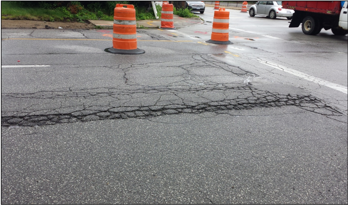
Photograph 9: East 22nd Street Pavement Distress
