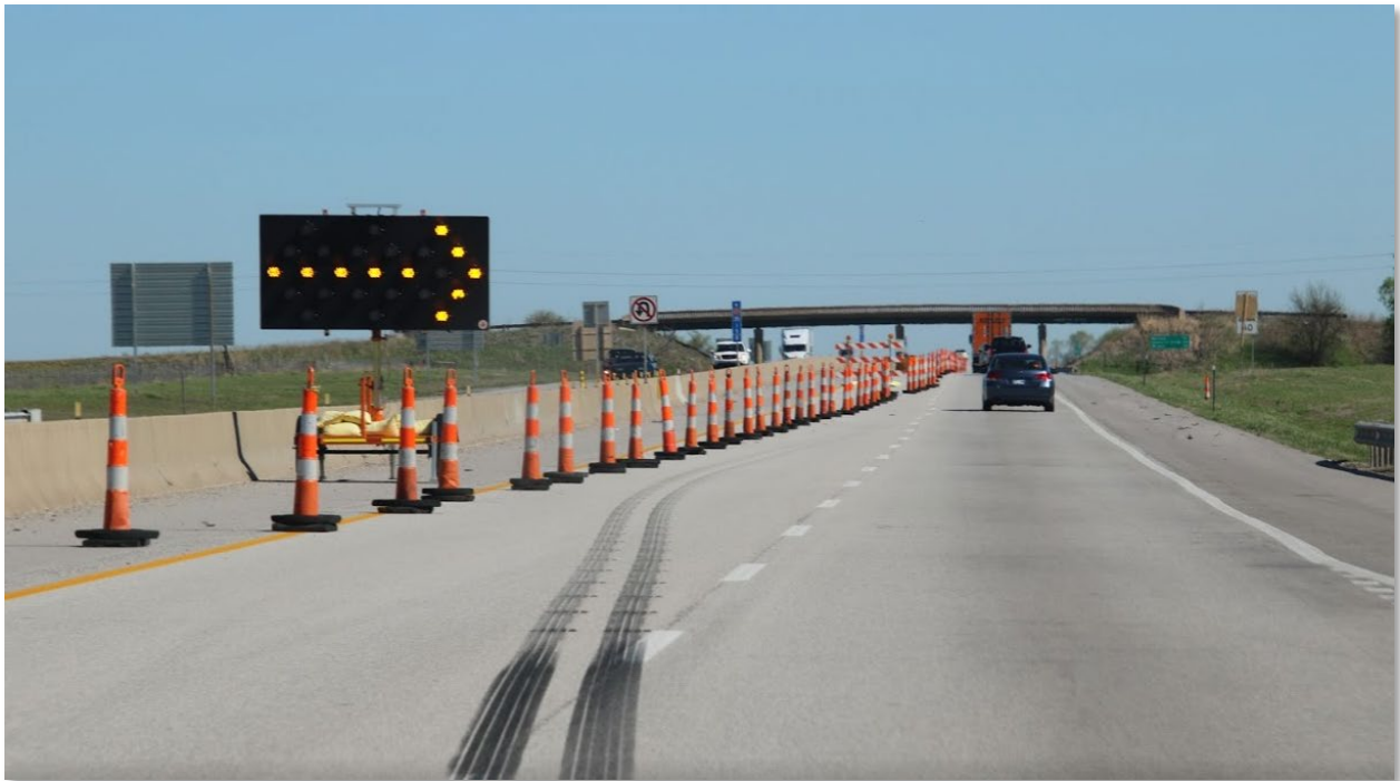
Figure 1: ODOT Connected Arrow Board
