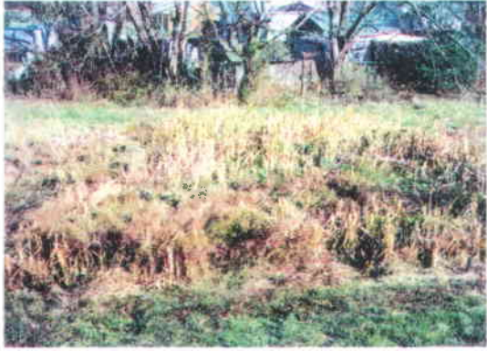
W23 WL4, emergent seep along embankment of US 52 in Wheelersburg.
