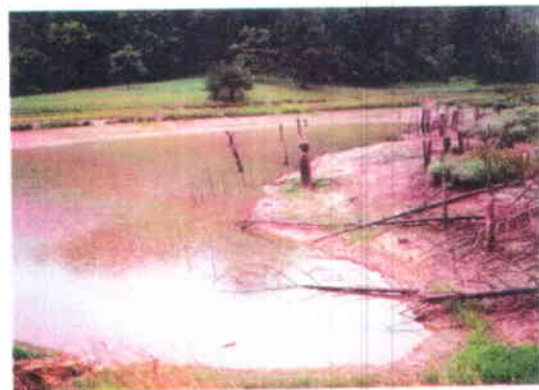
W8. Large pond drawn down due to embankment failure. Wetland vegetation developing along perimeter.
