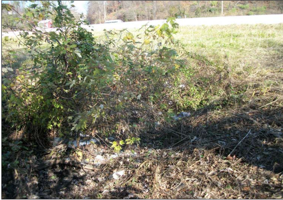
Photograph 319. Stormwater outlet pipe from US 52, facing north.
