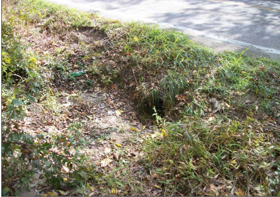
Photograph 253. Stream 39 culvert under SR 335 that drains to Little Scioto River, facing southeast.
