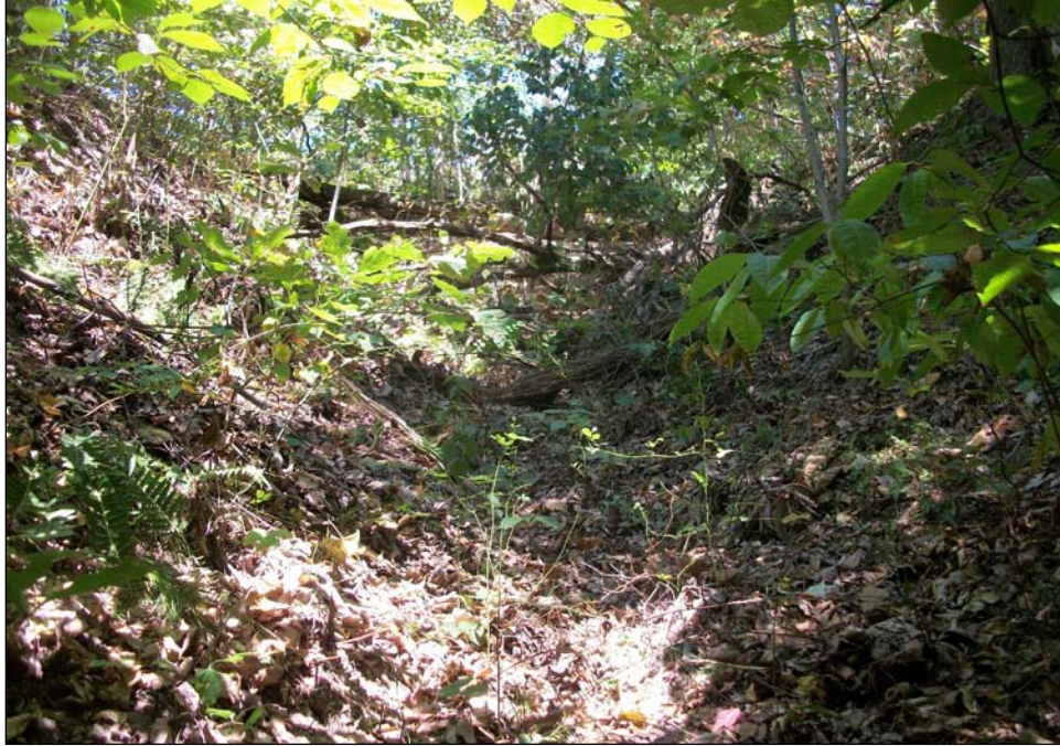
Photograph 165. Erosional feature upstream of Stream 28, facing northeast.
