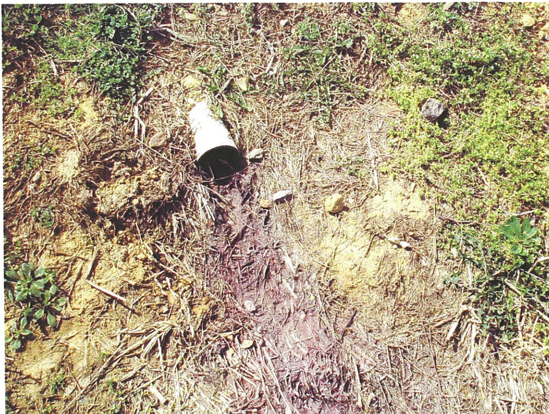
Photo 19. View looking at the area that the trench drains discharge onto the ground surface.
