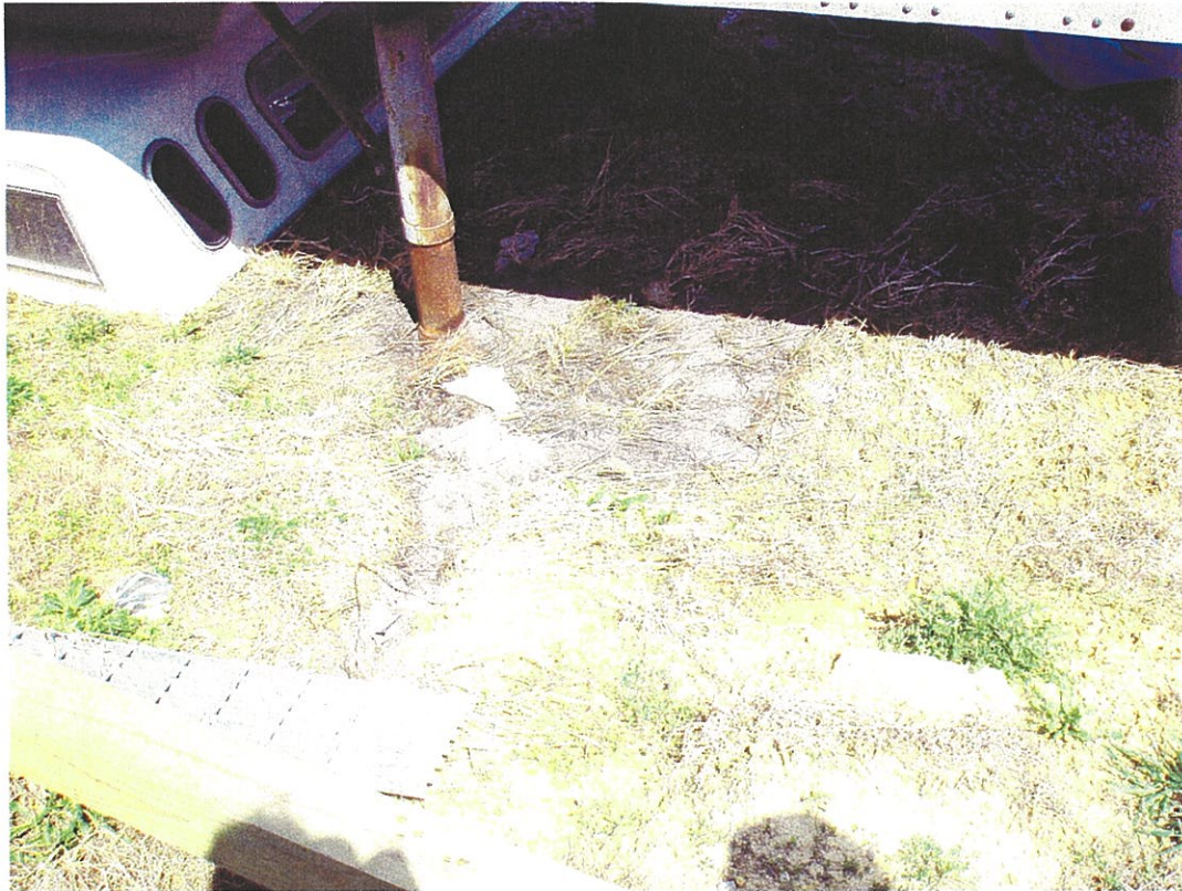
Photo 17. View looking at the area that the trench drains discharge onto the ground surface.
