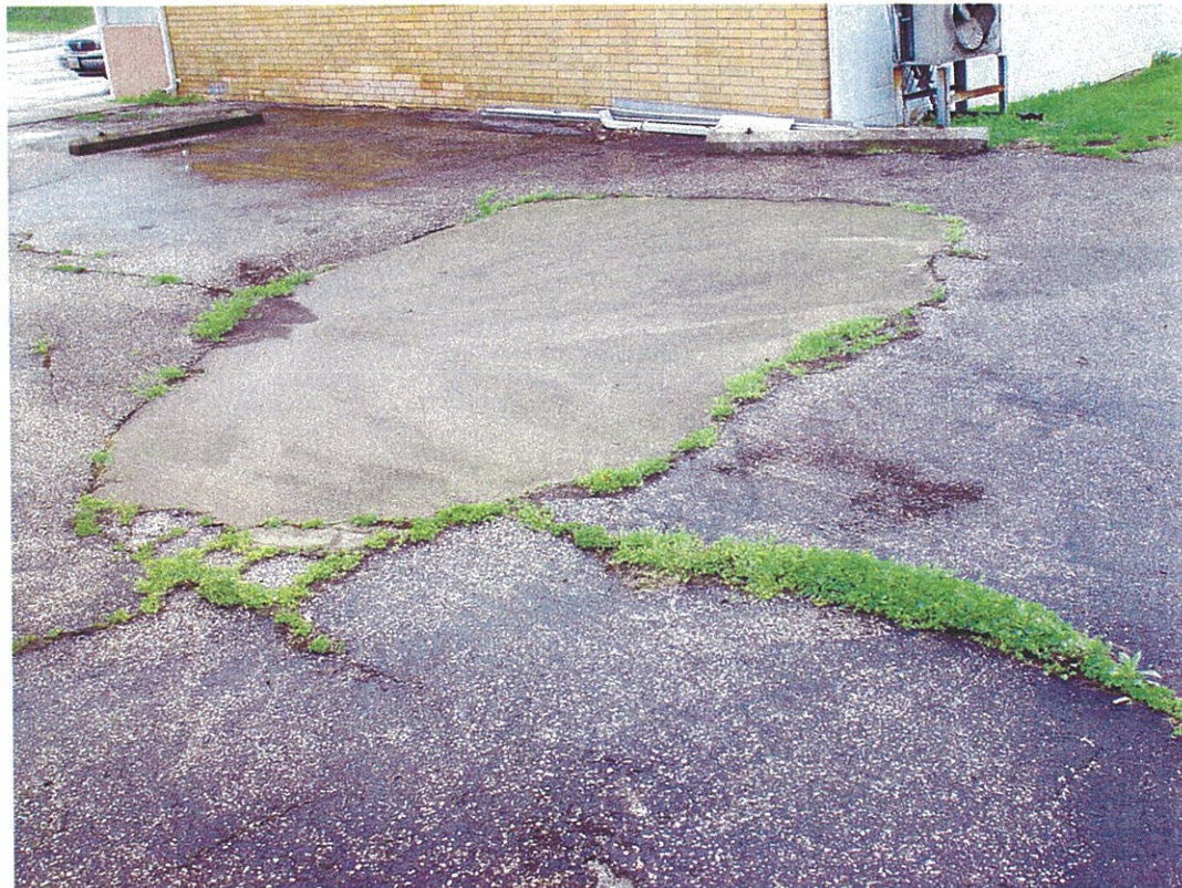
Photo 36. View of the patched pavement located on the eastern portion of the Harwood's gasoline station property.
