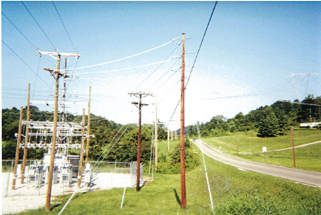
Photo 10. Overhead transmission lines and electrical/transmission facility. Rte. 728/Co. Road 28 (facing west).
