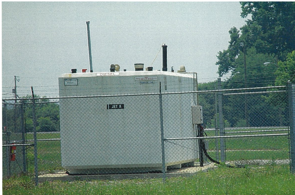
Photo 12. View of the AST located on the Scioto County Airport property.
