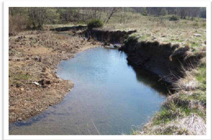
Photograph 4 (4-16-14). Candy Run East impairments include sedimentation, fecal coliform bacteria, and habitat modification. Work on the Candy Run East site will restore a natural channel and riparian corridor to this degraded stream.
