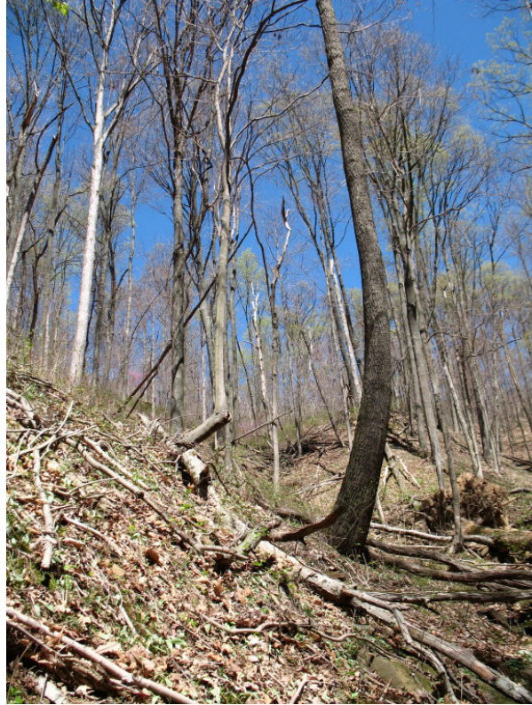
Photo 7. Indicators of slope instability, right of station 673+50.
