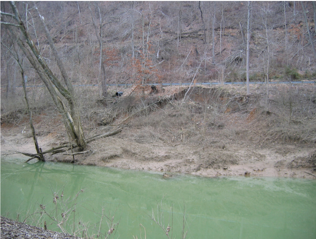
Photo 6. Landslide along SR 335.
