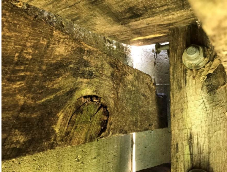
Picture # 5 - Failed south horizontal sidewalk support board at cantilever 1.
