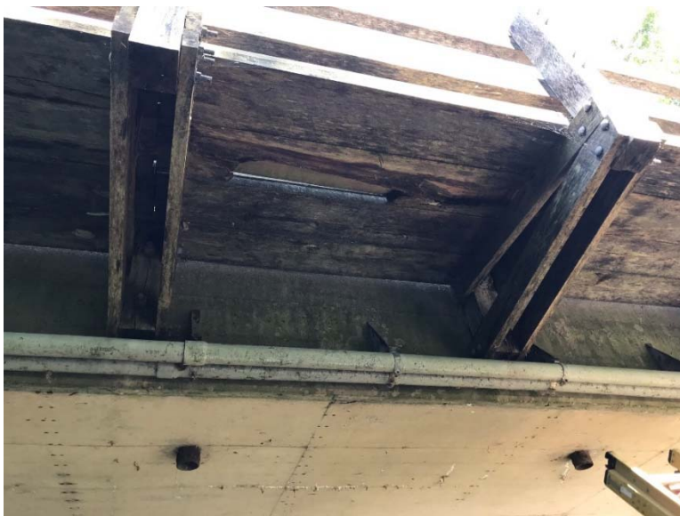
Picture # 2 - Hole in sidewalk plank in bay 4.
