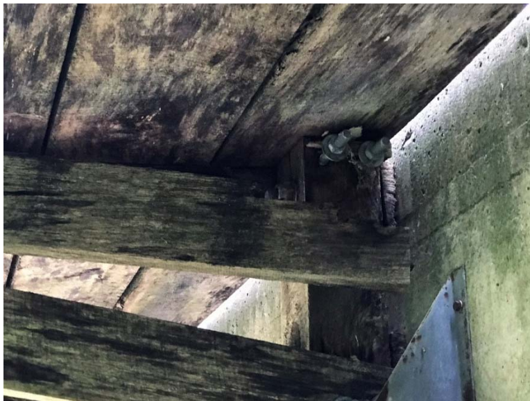
Picture # 6 - Failed north horizontal sidewalk support board at cantilever 13.
