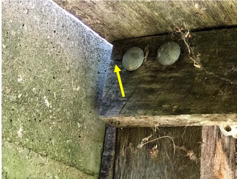
Picture # 3 - Split at connection bolts at cantilever 7.
