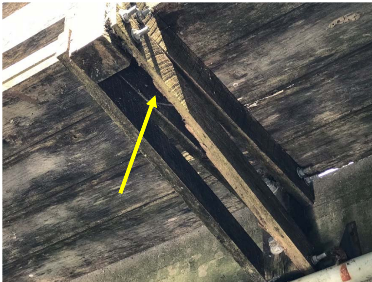
Picture # 4 - Heavy deterioration on north diagonal on cantilever 13.
