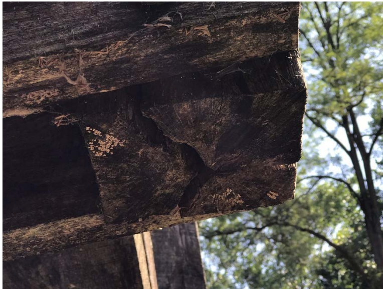
Picture # 9 - Large splits in bottom of post 7.
