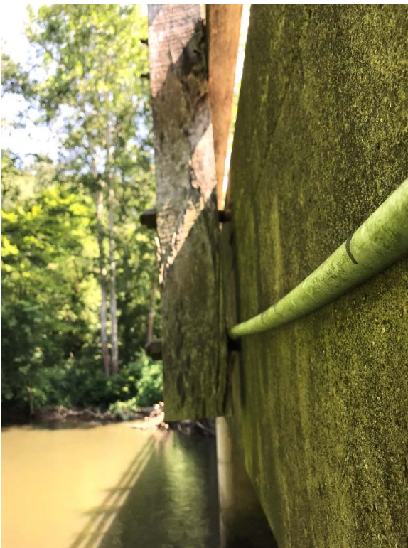
Picture # 10 - Typical gap between upstream railing post and slab. Note defunct conduit.
