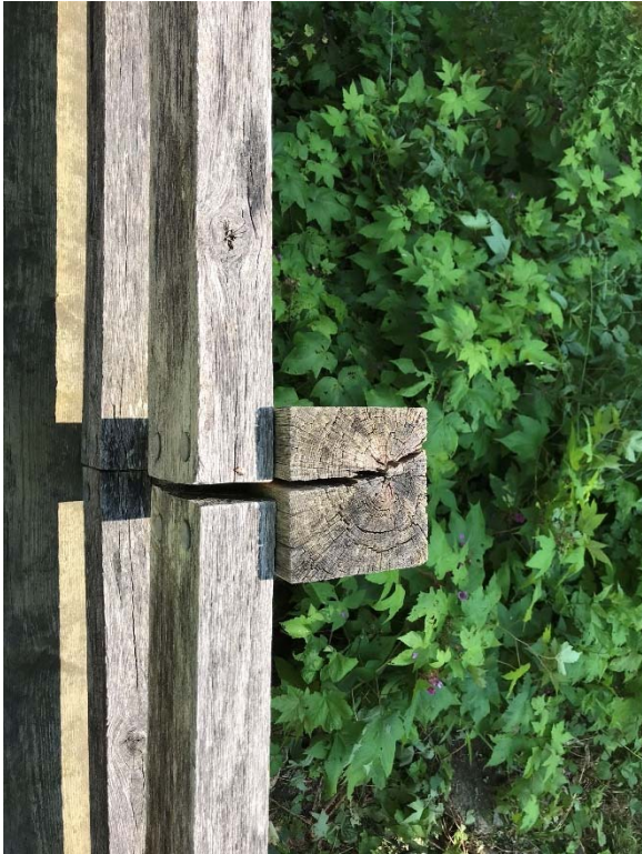
Picture # 8 - Split in top of post 2.
