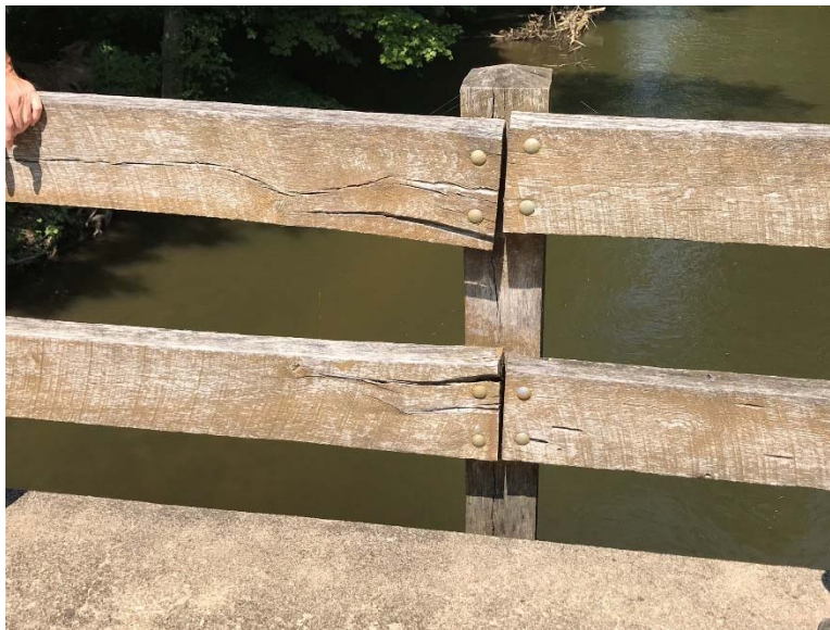
Picture # 12 - Typical cracked panels on upstream railing.
