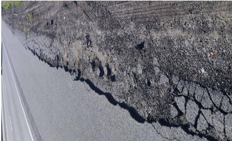
Photograph 7: Transverse and Longitudinal Cracking Along Project Ramps
