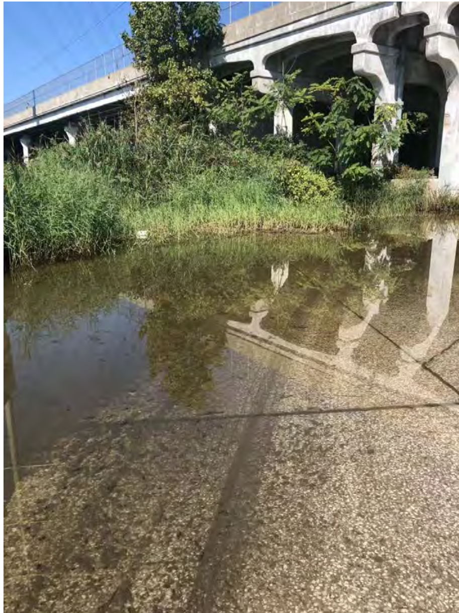
P14: Standing water observed under the bridge by the railroad
