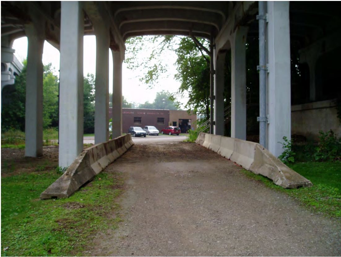
Barriers Placed by Cuyahoga County Engineer's Office to protect piers
