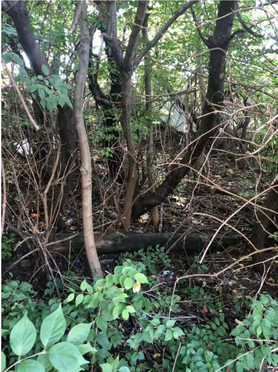
P8: Creep trees at the forward abutment embankment
