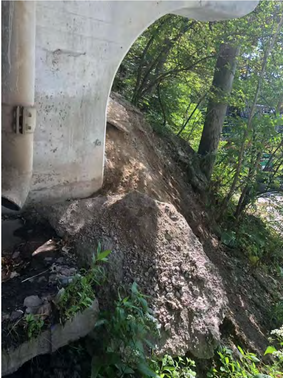
P7: Sloughy soil at the forward abutment embankment
