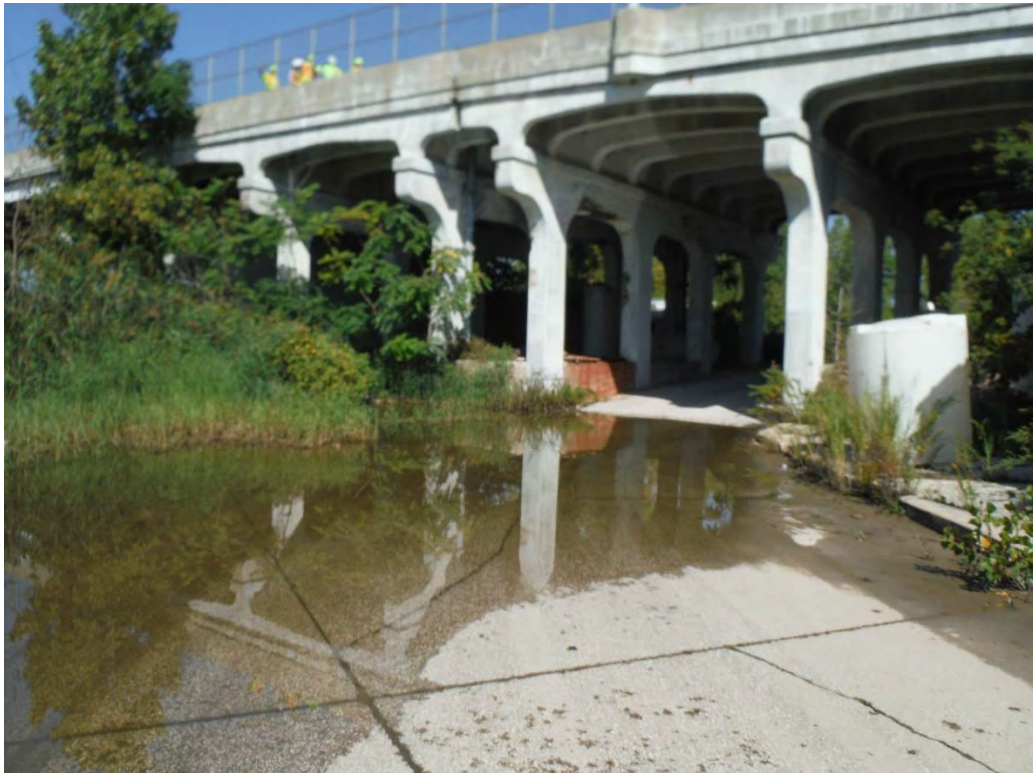
Figure 5. Flooding near Zone A Floodplain – Looking North
