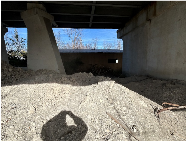
View of stockpiled material facing south with the building in the background.
