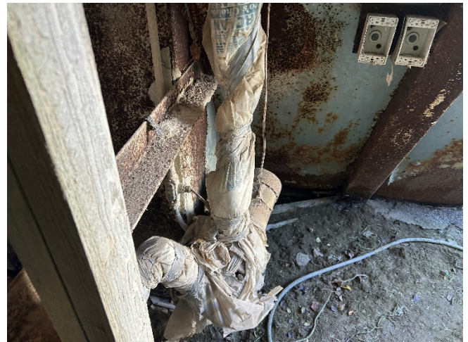
View of pipe wrap located in the building.
