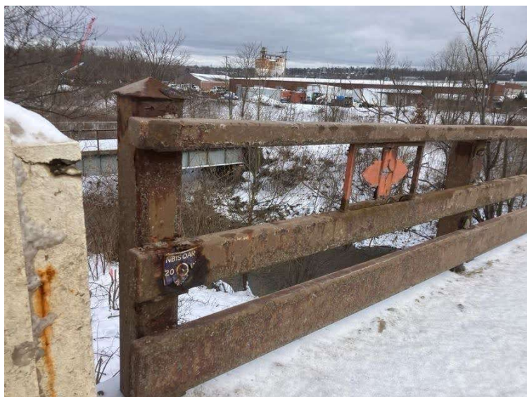
PHOTO 2 View of the metal railing. Samples were collected for the flaking paint and found to not contain ACM.
