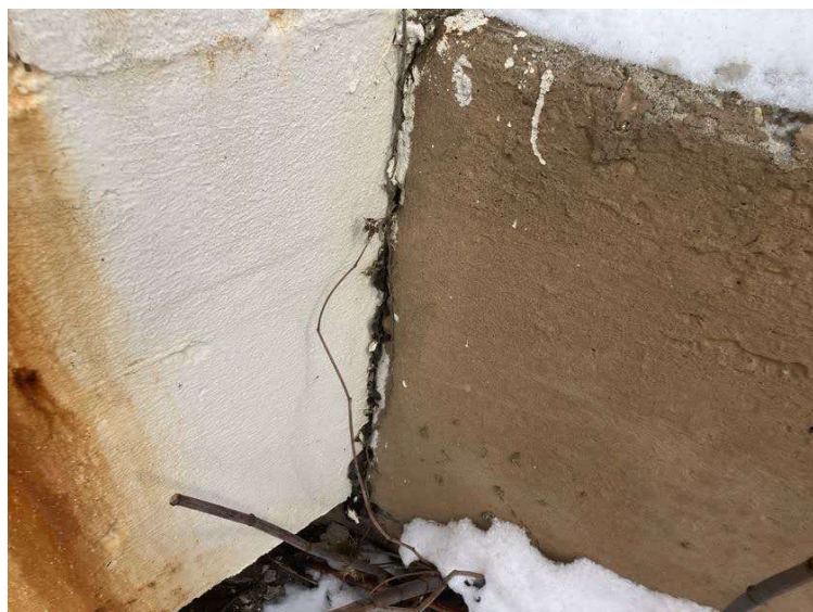
PHOTO 11 View of the expansion joint material where the wingwall and deck slab meet. Samples collected were ACM.
