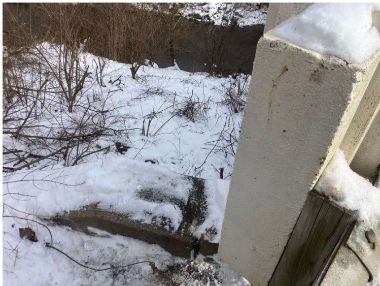
PHOTO 10 View of the top of the wingwall where the expansion joint was sampled. Sample results indicate it was ACM.
