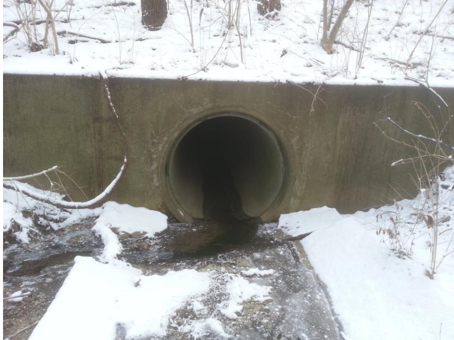
Photograph 5: View of corroded culvert.
