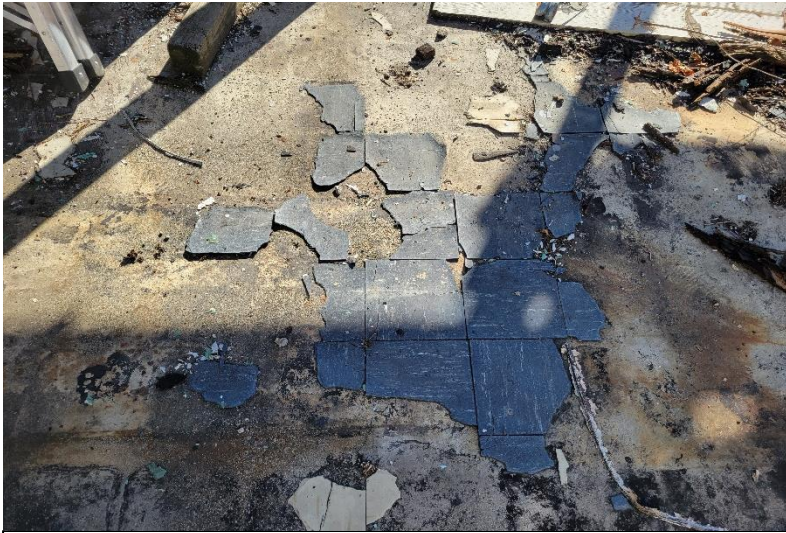
Photo 1 – View of asbestos-containing black floor tile in the concrete structure.
