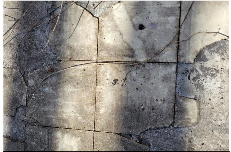
Photo 2 – View of asbestos-containing tan floor tile in concrete structure.
