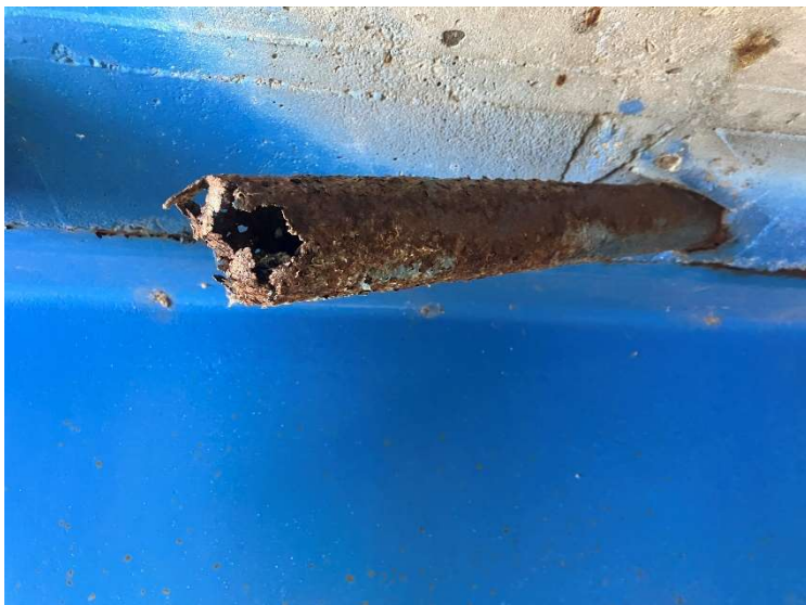
PHOTO 12 View of out of service small diameter metal conduit located underneath the southside of the structure. No wrapping, gasketing material, or other suspected ACM was observed.
