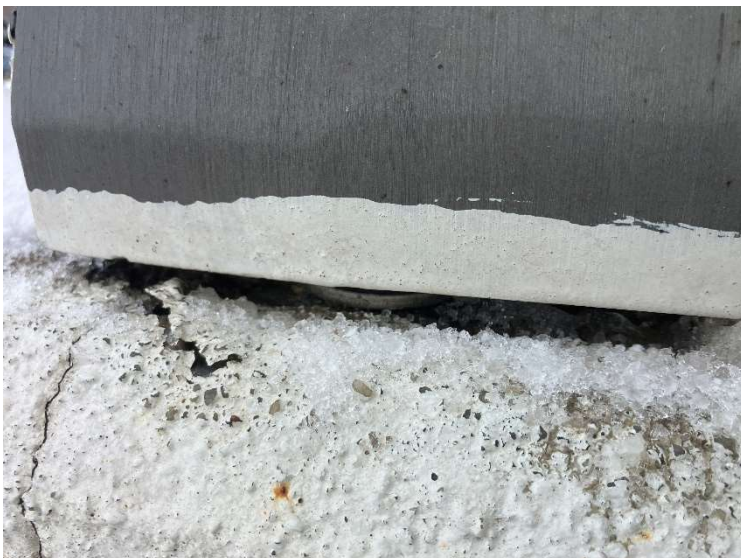
PHOTO 3 A close-up view of one of the steel parapet railing mounting brackets. No caulking, gasketing, or other suspected ACM was observed beneath the base.
