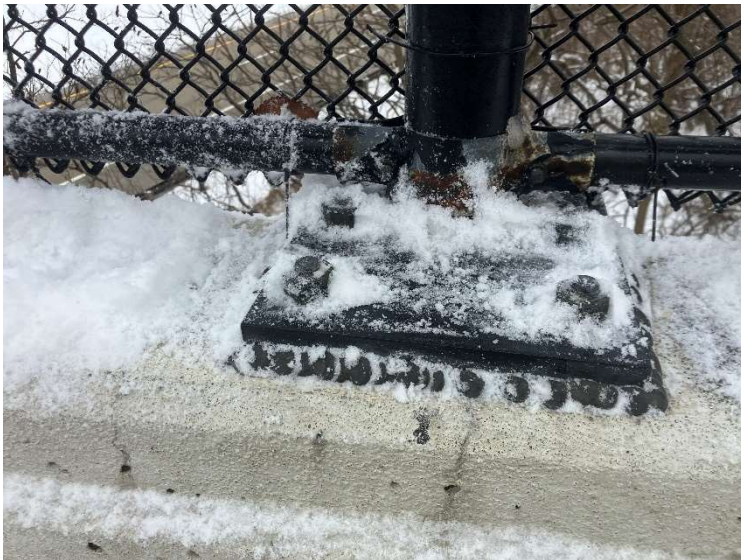
PHOTO 2 View of the vandal fence base with caulking material around the base. Samples were collected and found to not contain ACM.
