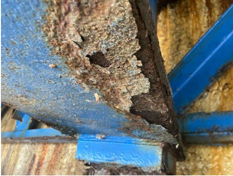
PHOTO 10 View of corroded and peeling paint on steel girder. Samples were collected and found to not contain ACM.
