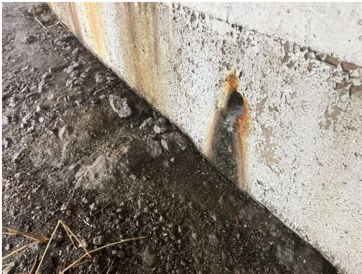
PHOTO 11 View of peeling curing sealer on concrete abutment wall. Samples were collected and found to not contain ACM.
