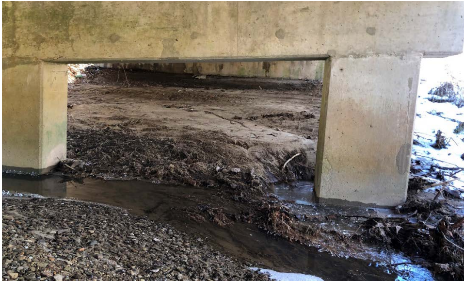
Photograph 5: Scour Observed at Western Pier
