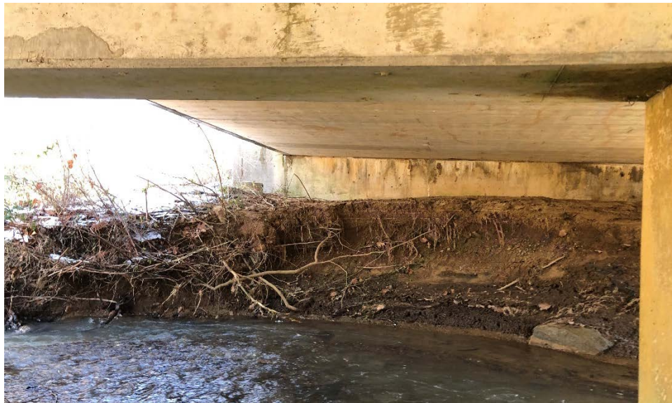
Photograph 4: Eastern Spill-through Slope and Observed Erosion
