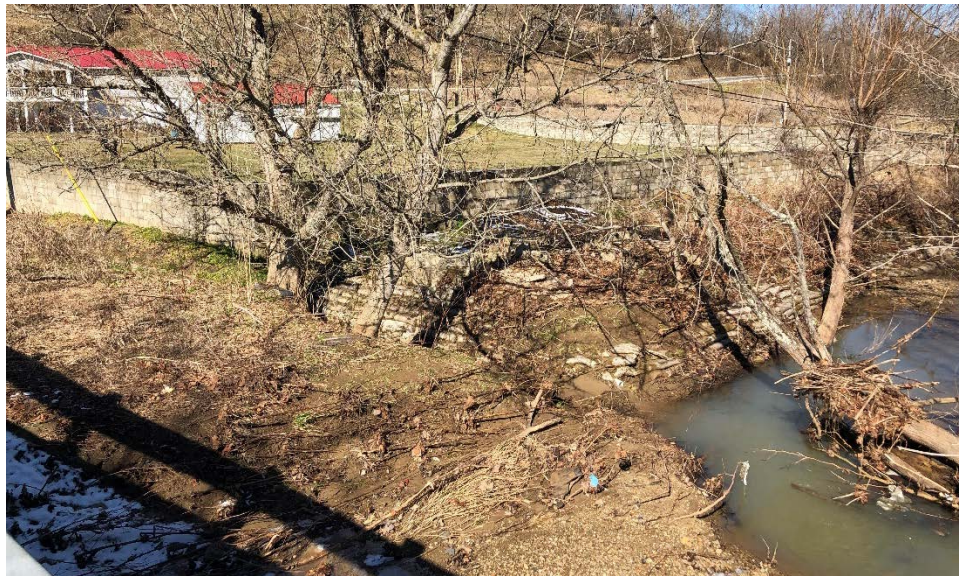
Photograph 2: Northwestern Bank of Creek Reinforced with Sandbags
