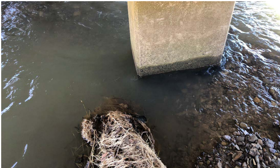
Photograph 6: Scour Observed at Eastern Pier
