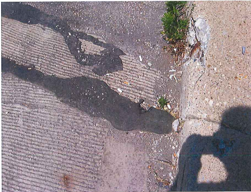
Photograph 4: Bridge MOT-CR-074-0.65, Roadway Expansion Joint
