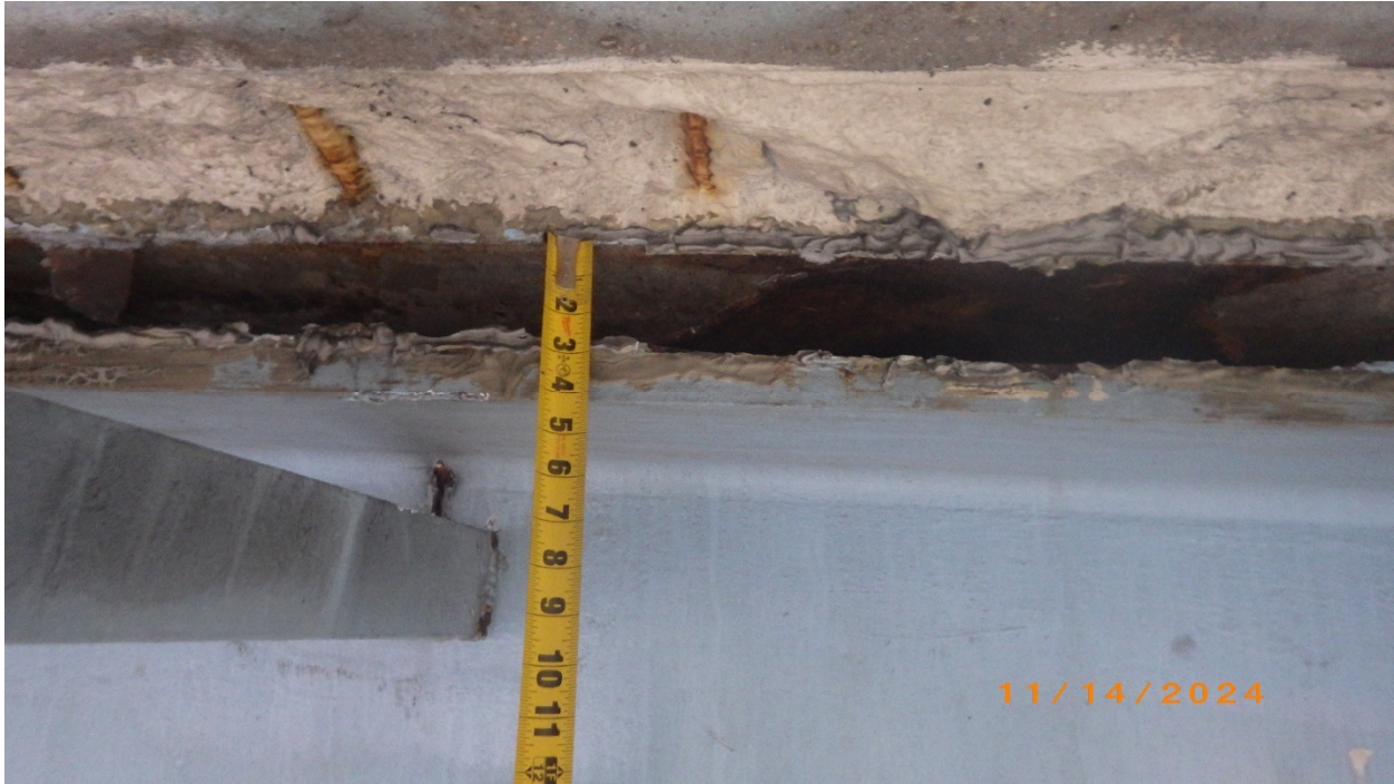
Photo # 13 – Beam 1, inside of top flange, separation from haunch at Crossframe 5
