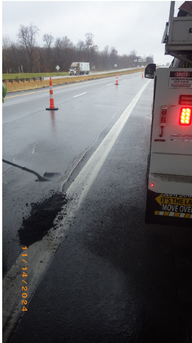
Photo # 40 – Pavement gouge in Westbound driving lane
