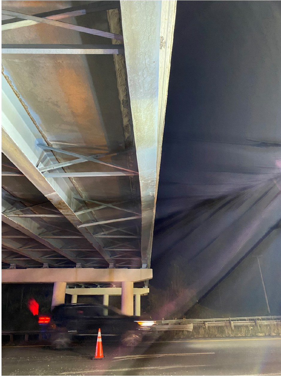
Photo # 1 - Span 3 Beams 1 and 2, looking south, immediately following impact
