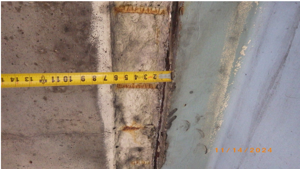
Photo # 39 – Existing spall from prior incidents, inside of Beam 1 top flange, shown near point of impact
