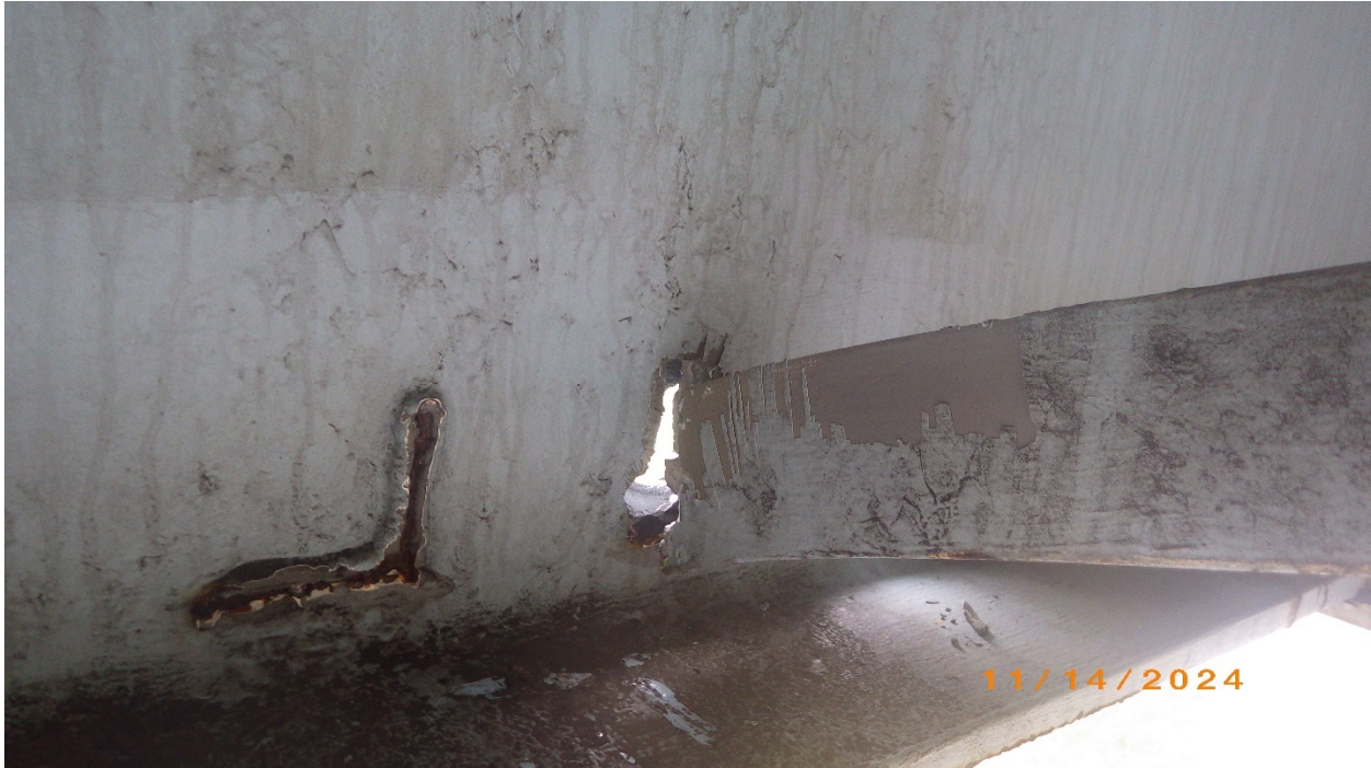
Photo # 38 – Crossframe 7 at Beam 1. Note full tearout of the web at the diagonal weld
