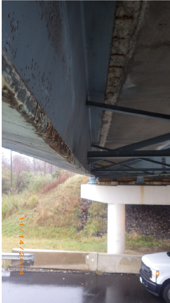
Photo # 7 - Beam 1, bottom flange, looking North from point of impact
