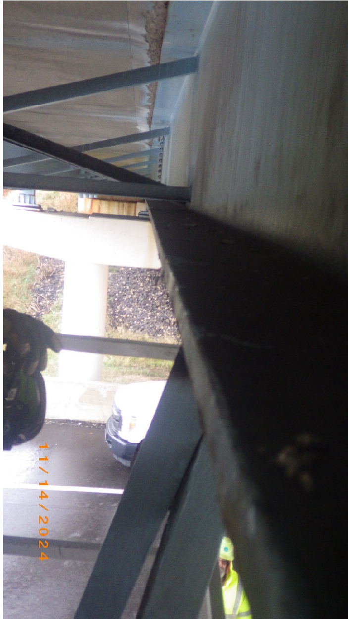
Photo # 22: Beam 2, looking North from point of impact. Note spalling
