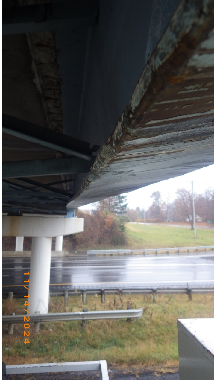
Photo # 6 - Beam 1, bottom flange, looking South from point of impact
