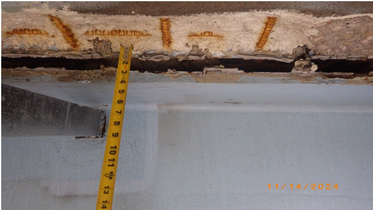
Photo # 12 – Beam 1, inside of top flange, separation from haunch at Crossframe 3
