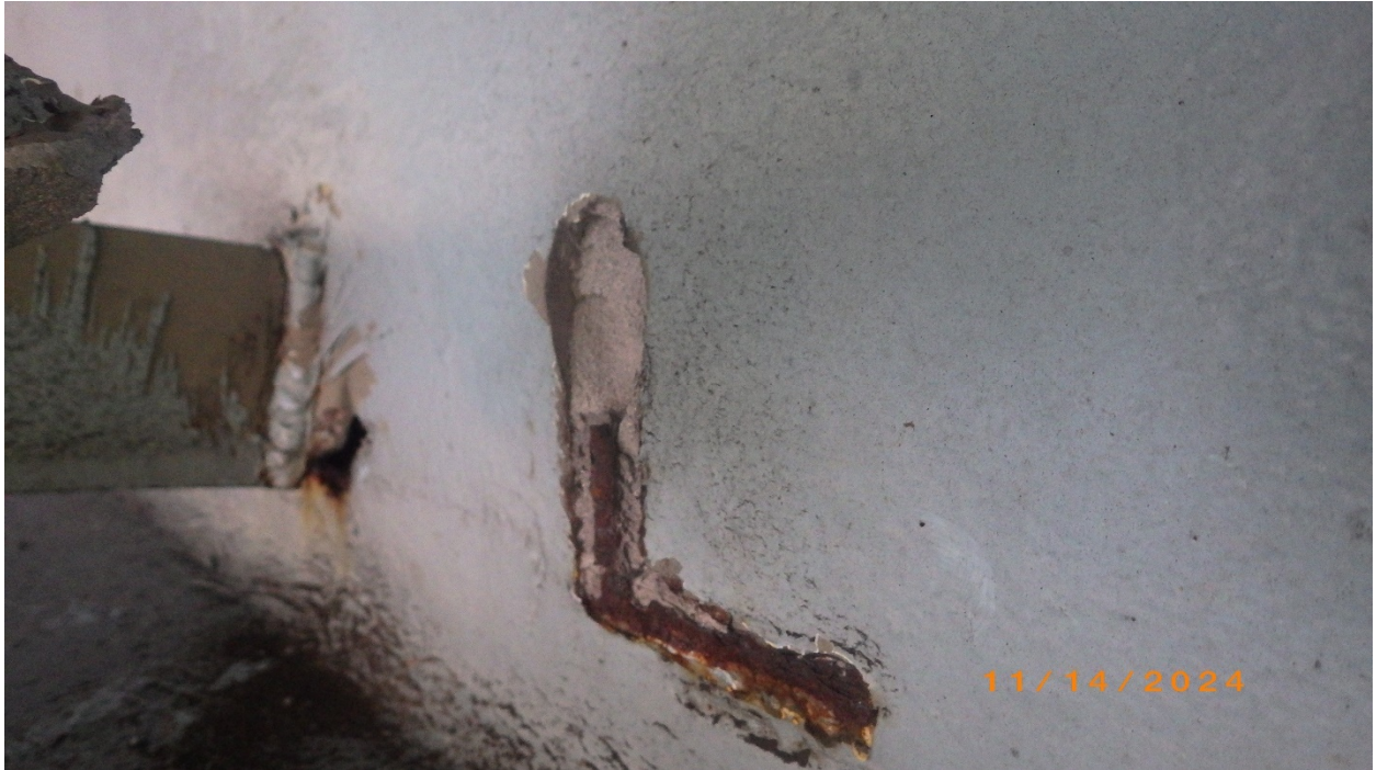
Photo # 28 – Crossframe 4 at Beam 1, lower diagonal weld. Note ~ 1/4" deep tearout of web material
