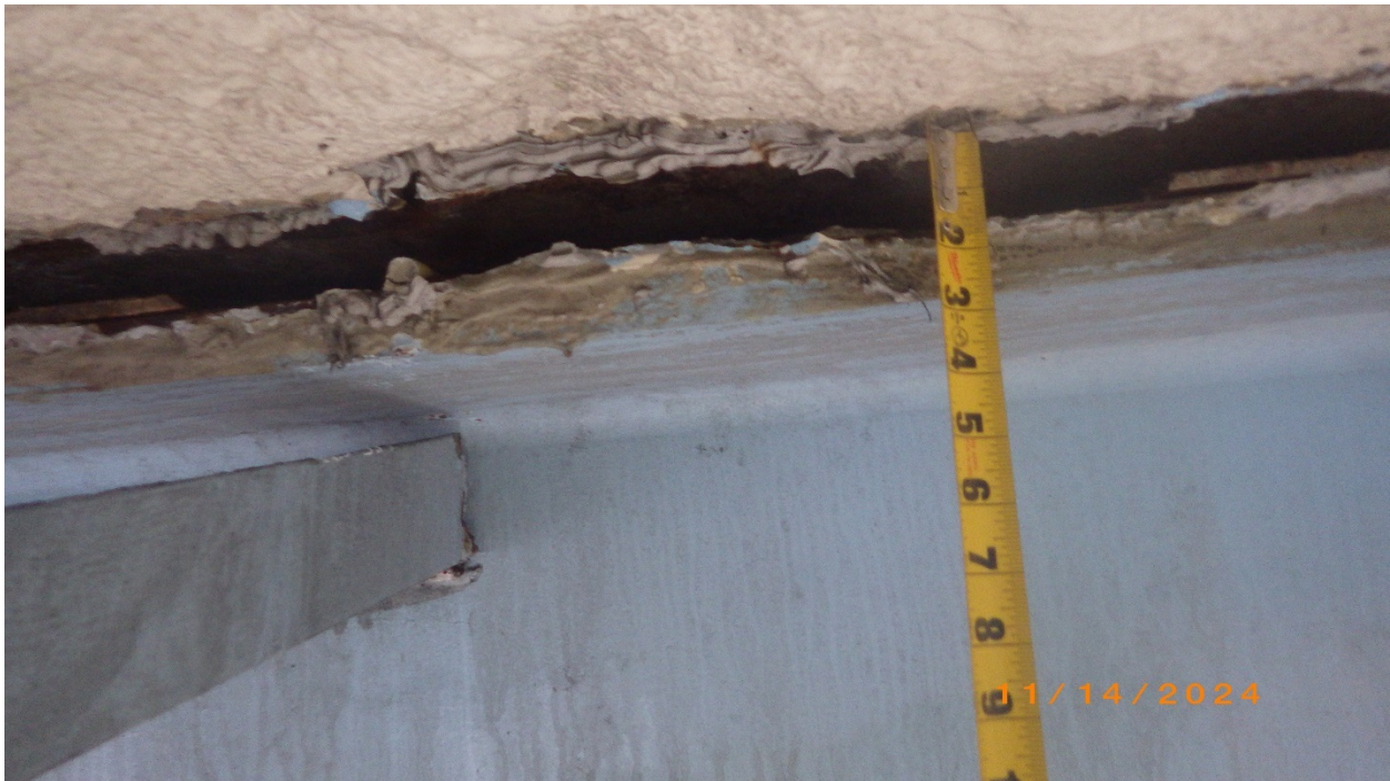
Photo # 14 – Beam 1, inside of top flange, separation from haunch at Crossframe 6
