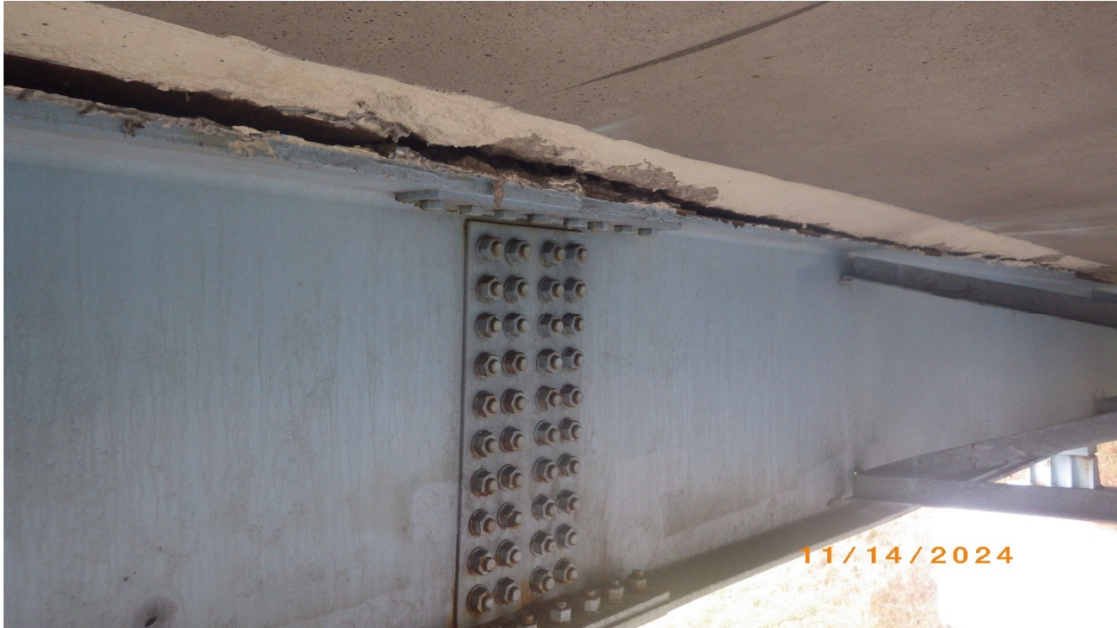
Photo # 15 – Beam 1 Span 3 Splice Plate. Note fresh spalling
