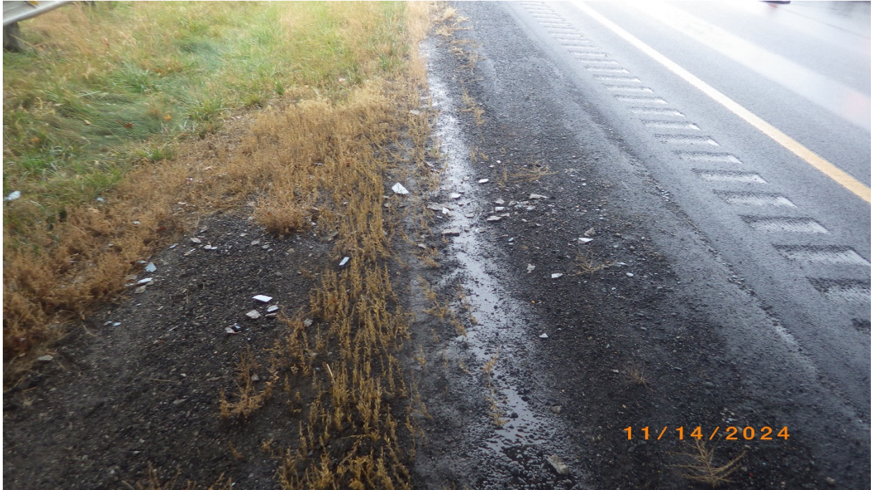
Photo # 19 – Fresh spalling on shoulder, South side of Westbound roadway
