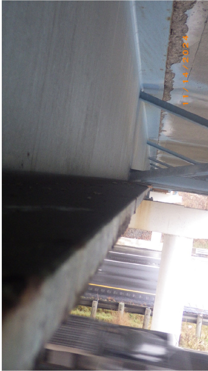
Photo # 21 – Beam 2, looking South from point of impact. Note spalling
