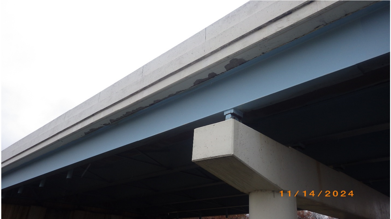
Photo # 17 – Span 3, Beam 1, outside, looking South. Note spalling
