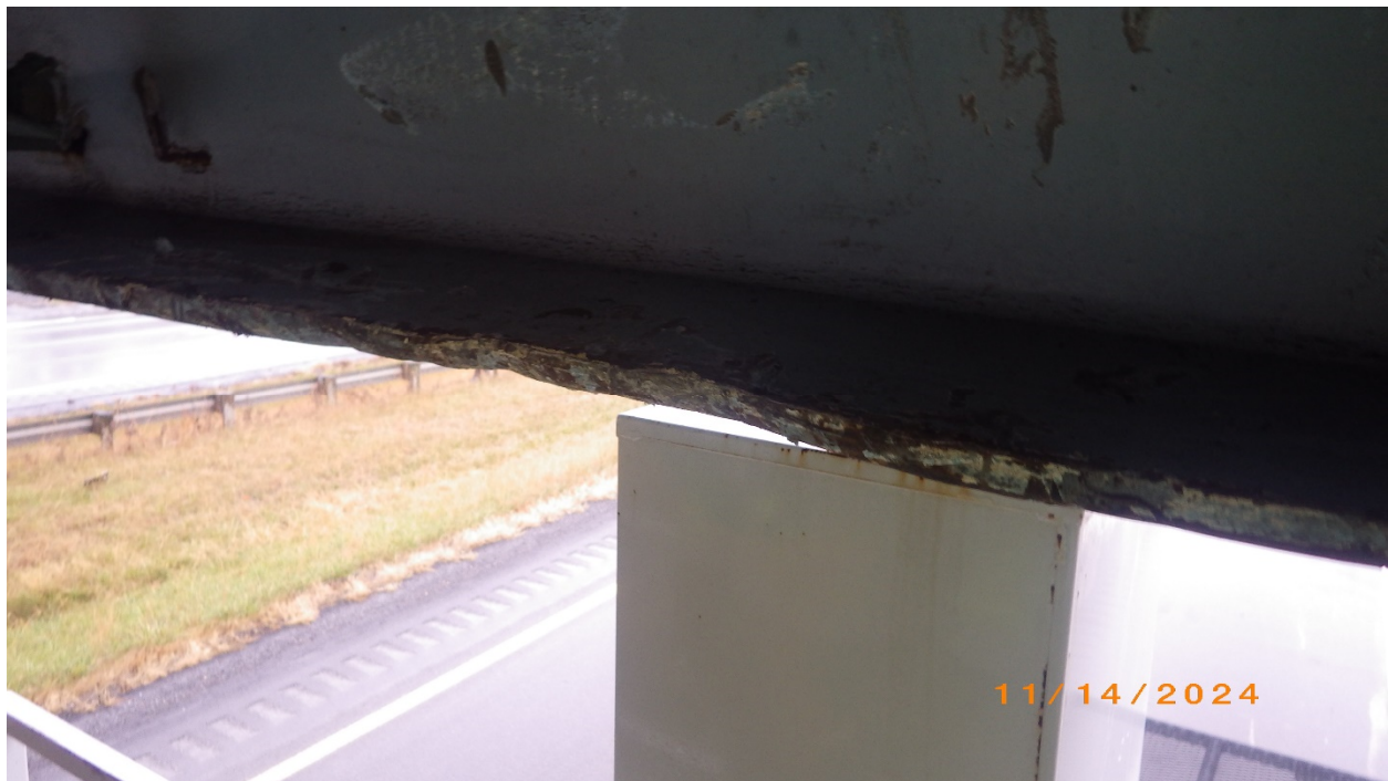
Photo # 5 - Beam 1, bottom flange condition at point of impact
