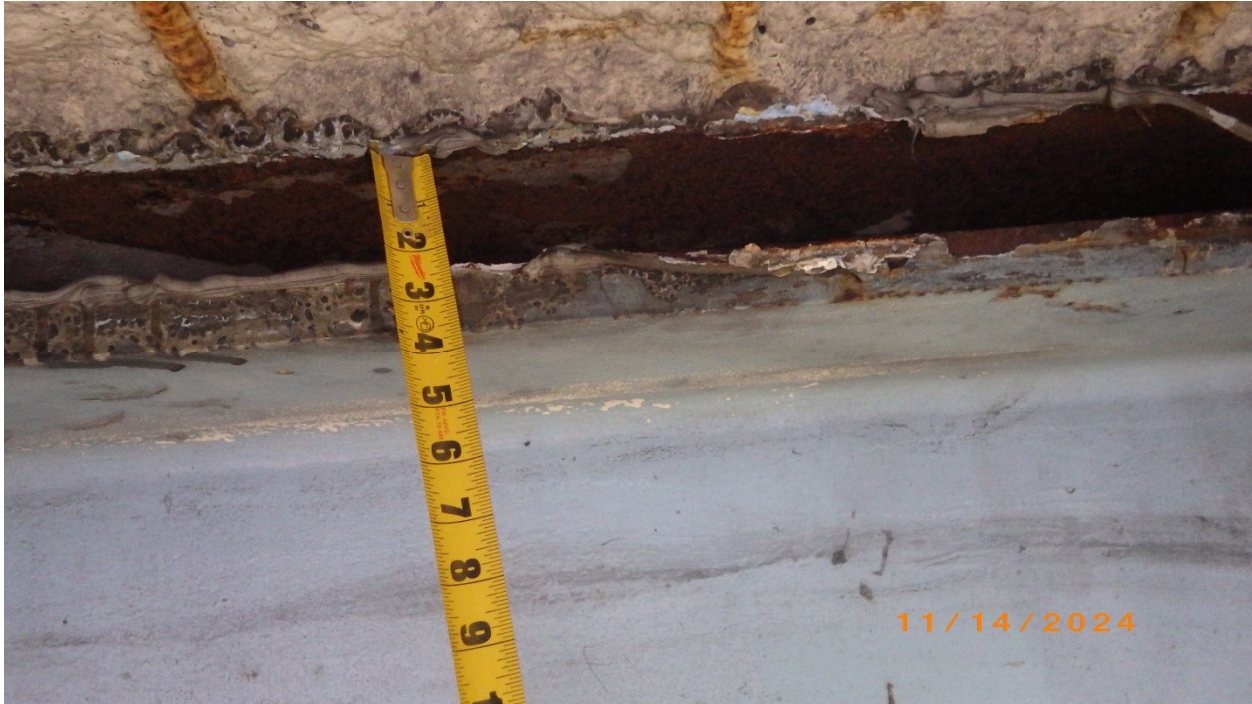
Photo # 11 – Beam 1, inside of top flange, separation from haunch at point of impact
