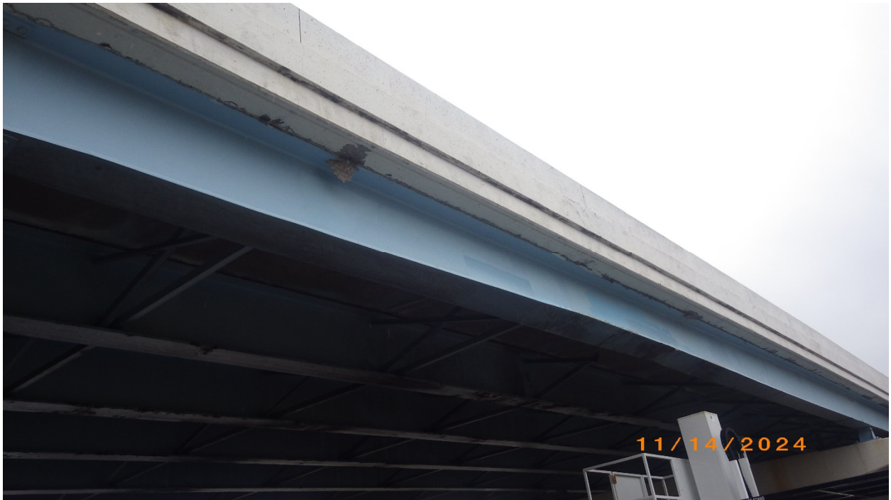
Photo # 18 – Span 3, Beam 1, outside, looking North. Note spalling. The hanging spall was removed by ODOT forces
