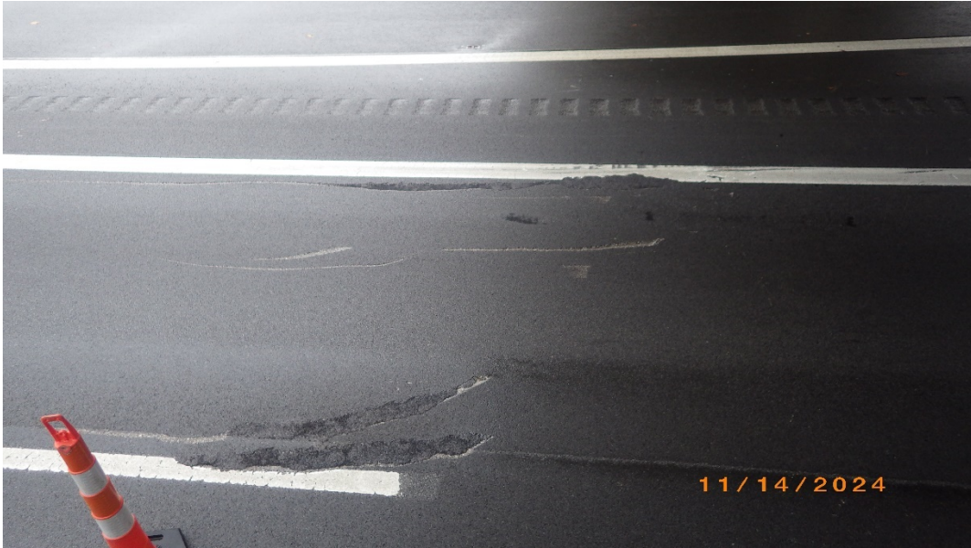
Photo # 41 – Pavement gouges in Westbound driving lane, filled with cold patch asphalt
