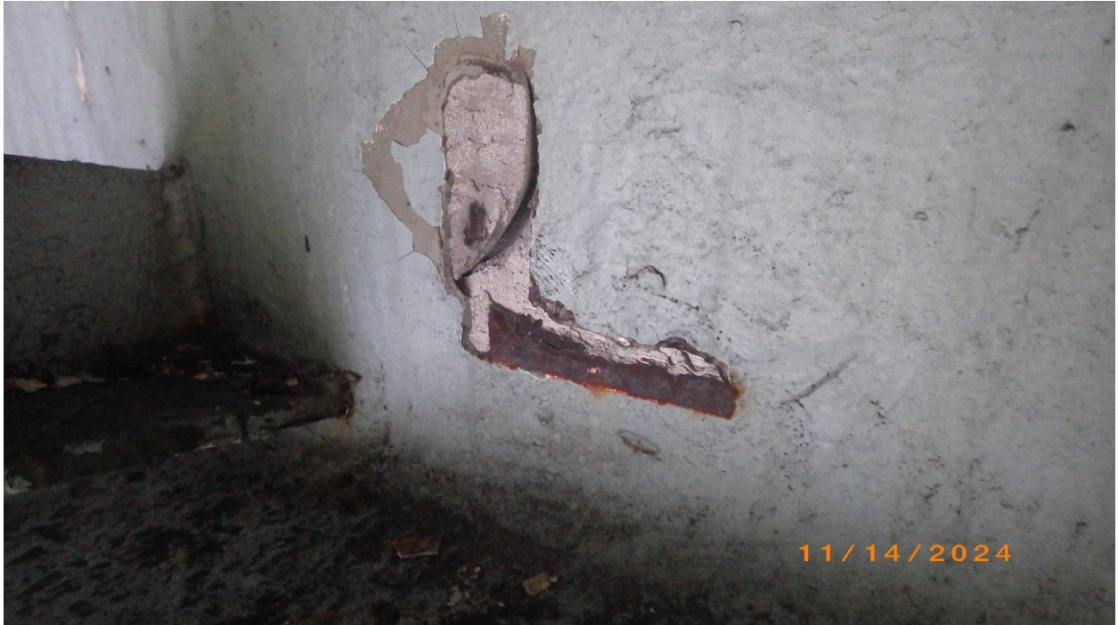
Photo # 30 – Crossframe 4 at Beam 2, lower horizontal weld. Note tearout of web material
