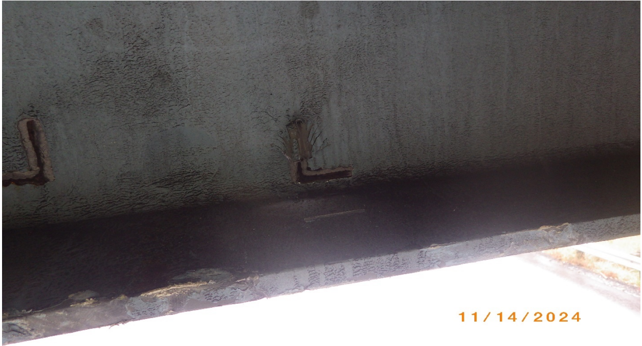
Photo # 32 – Crossframe 5 at Beam 1, lower welds. Note tearout of web material at horizontal member weld
