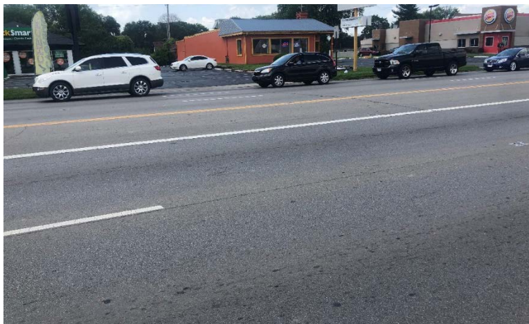
Photograph 2: Overall Pavement condition of N Bridge St Between N Plaza Blvd and Pawnee Rd
