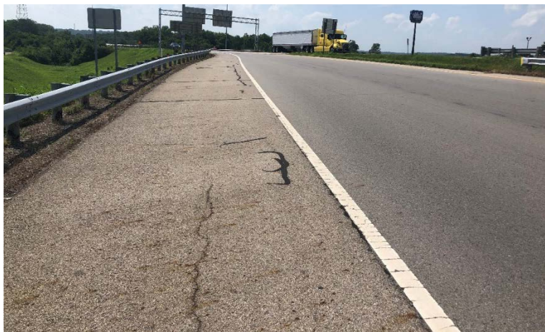
Photograph 4: Overall Pavement condition of Ramp US-35 EB
