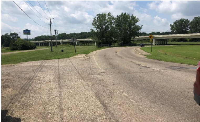
Photograph 6: Overall Pavement condition of Stewart Street
