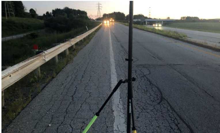
Photograph 5: Pavement condition of IR-77 NB ramp from Ghent Road (Ramp M)
