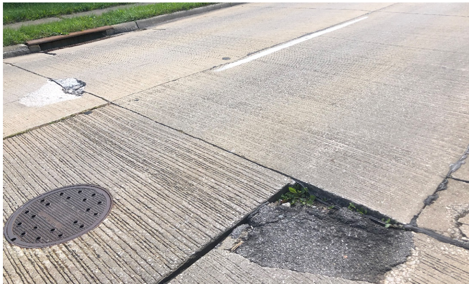
Photograph 8: Pavement Condition of Fountain Street
