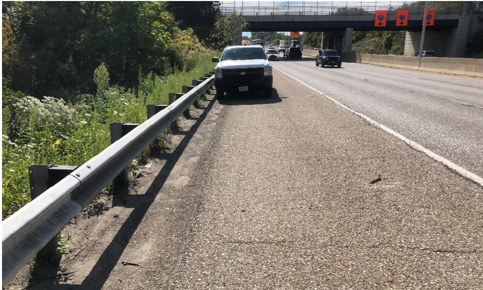
Photograph 5: Overall Pavement Condition of SR-8
