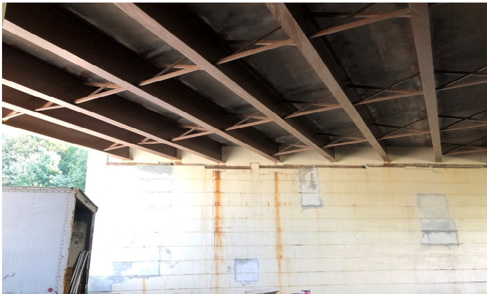
Photograph 3: Signs of Infiltration at Expansion Joints
