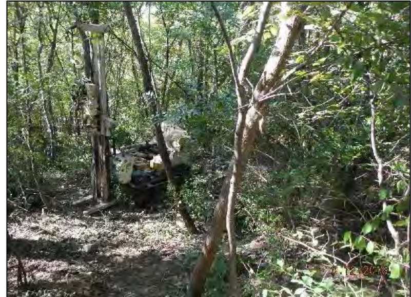
Photo 14 - View of Geoprobe drill rig set up at boring EB-4, facing south.
