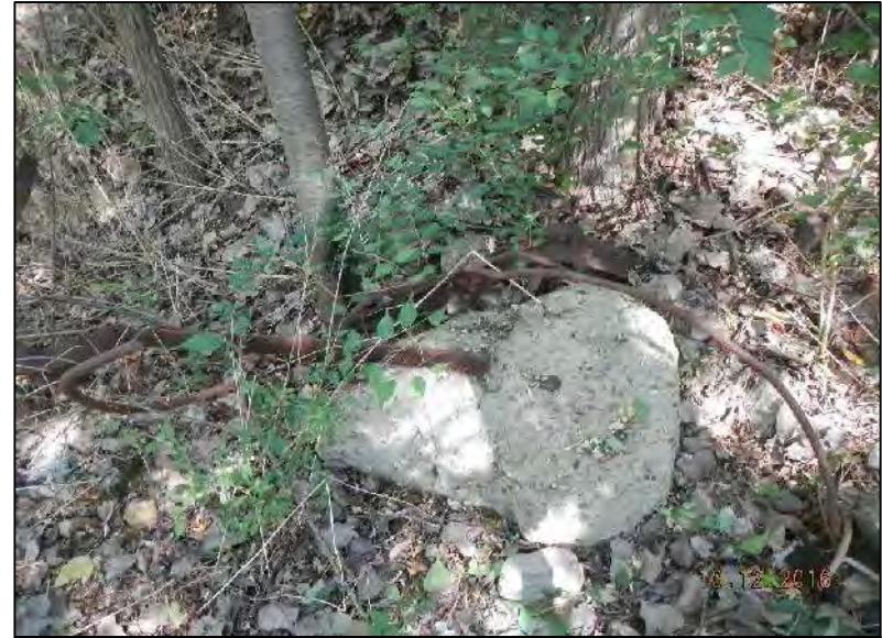
Photo 34 – Typical view of rebar and concrete throughout the wooded portions of the project site.
