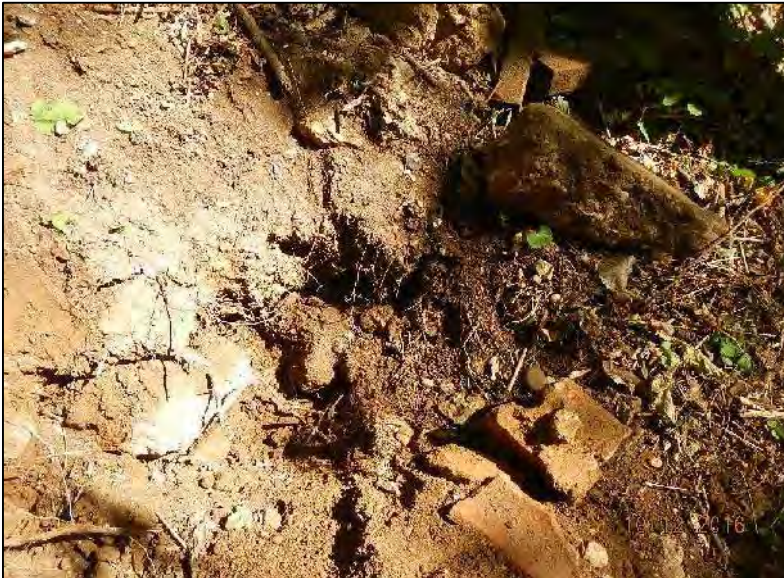
Photo 31 - Close up view of fill materials at HS-1 (concrete, rock and brick boulders and scrap metal).
