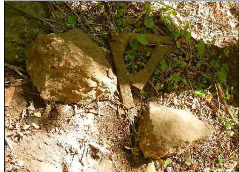
Photo 32 - Another close up view of fill materials at HS-1 (concrete, rock and brick boulders and scrap metal).
