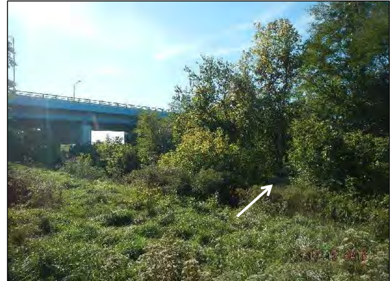
Photo 10 - View of Geoprobe drill rig set up at boring EB-3, facing southeast.
