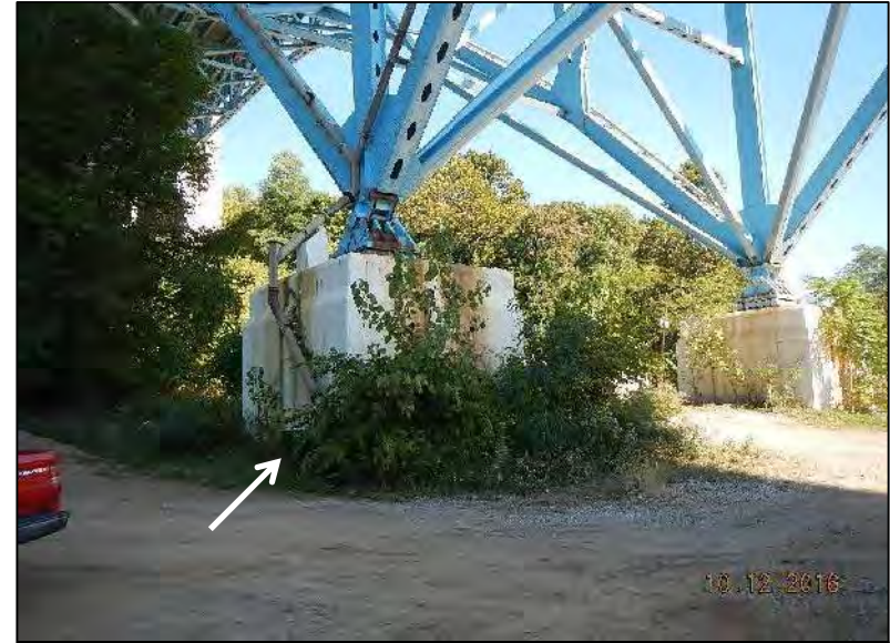
Photo 38 – View of the drum containing non-hazardous soil cuttings and decontamination rinse water located at the bridge pier foundation, awaiting characterization for proper disposal.
