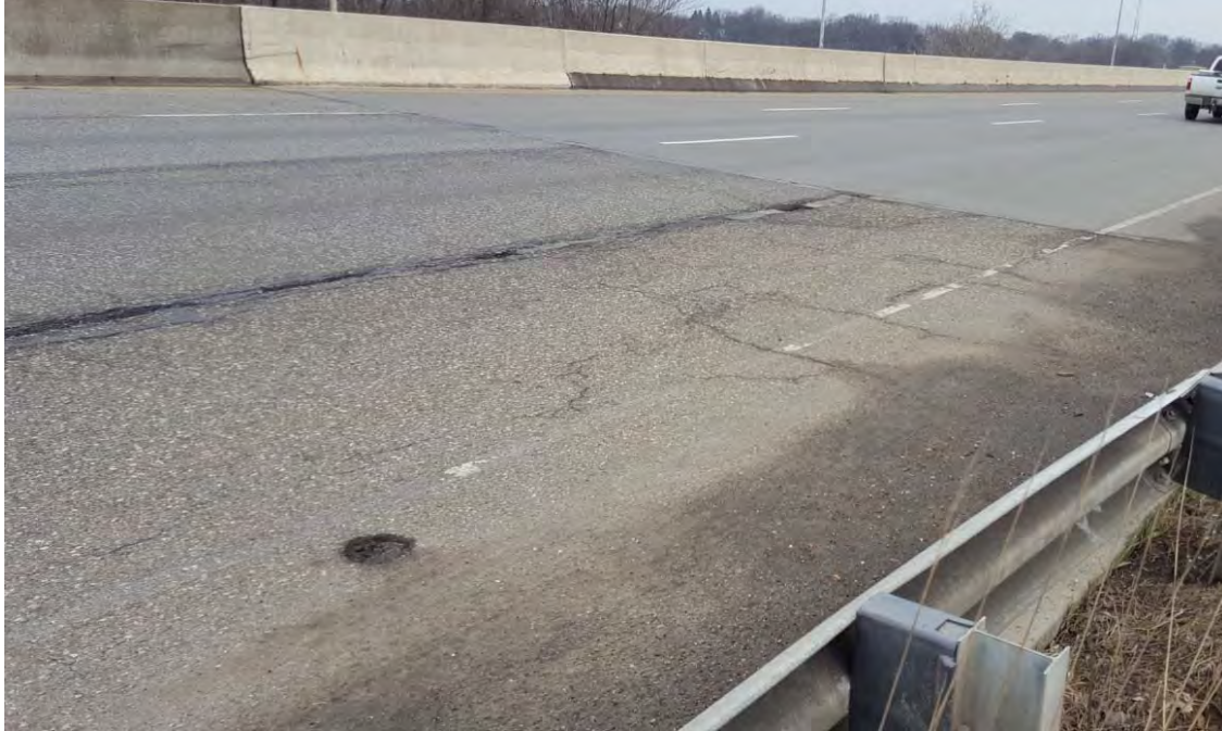
Photograph 6: Medium to high severity longitudinal cracking along SR-8 NB
