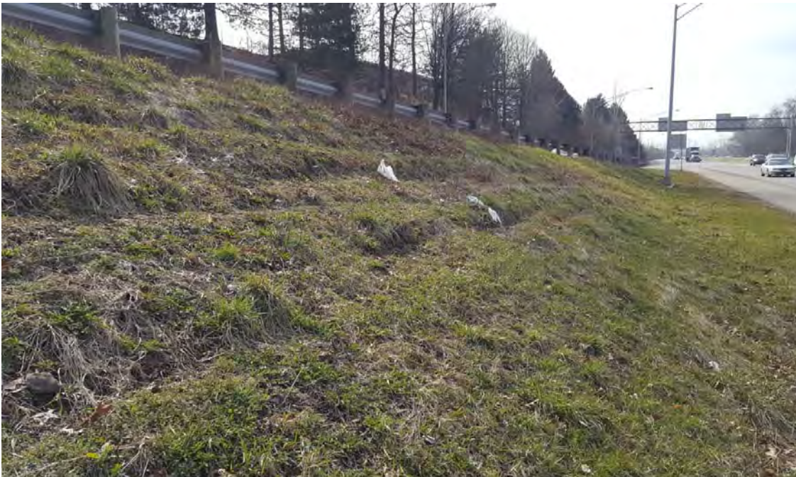
Photograph 3: Minor scarps on embankment slope at SR-8 NB exit ramp to E. Glenwood Ave
