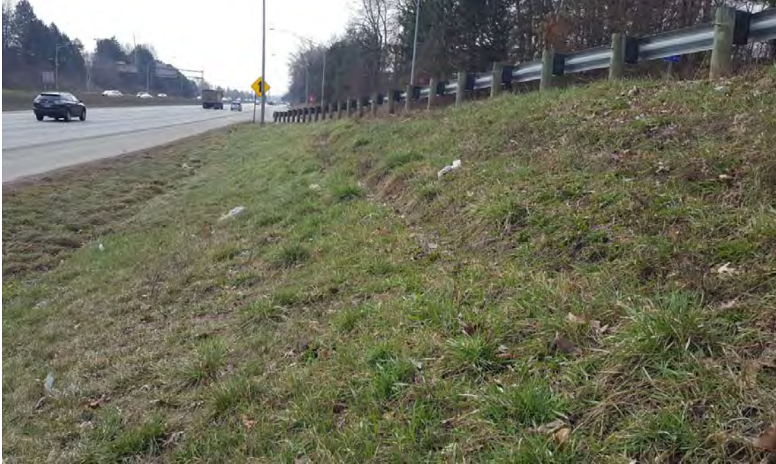
Photograph 4: Minor scarps on embankment slope at SR-8 SB entrance ramp from E. Glenwood Ave
