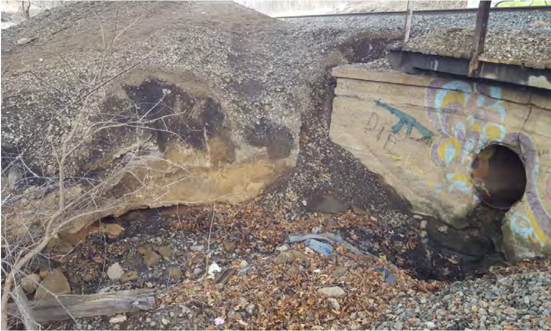
Photograph 2: Sign of erosion at storm sewer outlet under south side of existing bridge (2 of 2)
