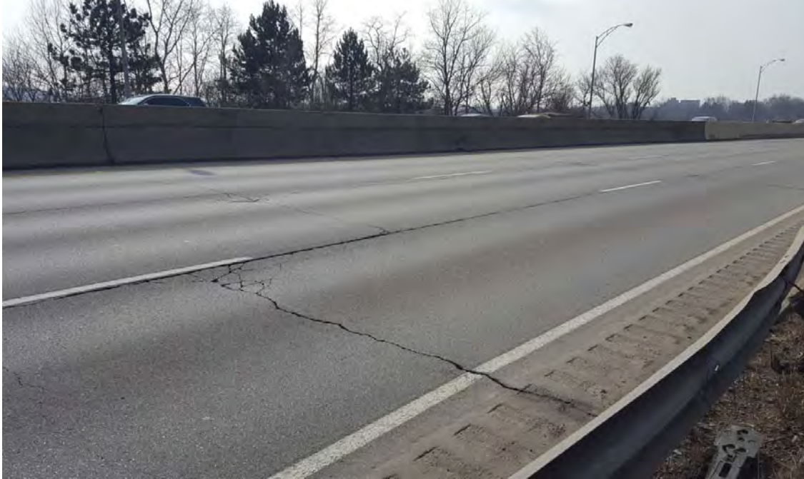
Photograph 8: Medium severity thermal cracking along SR-8 SB
