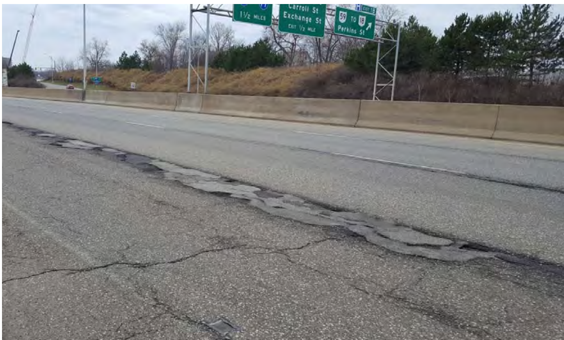
Photograph 5: High severity longitudinal cracking and pothole patching along SR-8 NB
