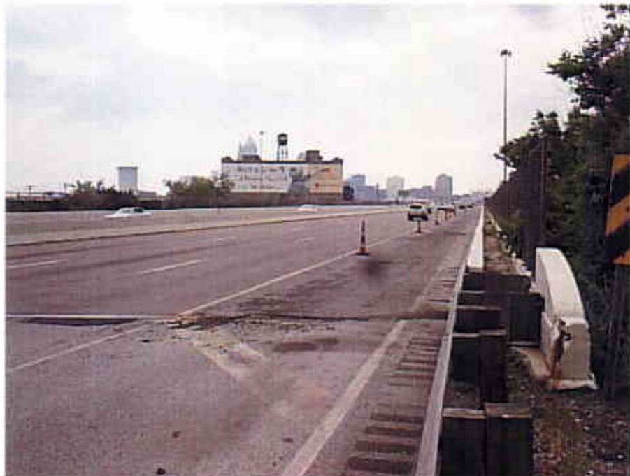
Photograph 28 View Looking North at the Top of the East Bound Lanes of the Interstate 90 Innerbelt Bridge over the Cuyahoga River (CUY-90-15.24)
