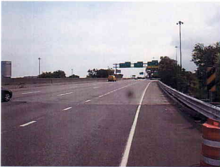
Photograph 24 View Looking East at the Top of the East Bound Lanes of the Interstate 90 Bridge over East 9 th Street (CUY-90-1628R)
