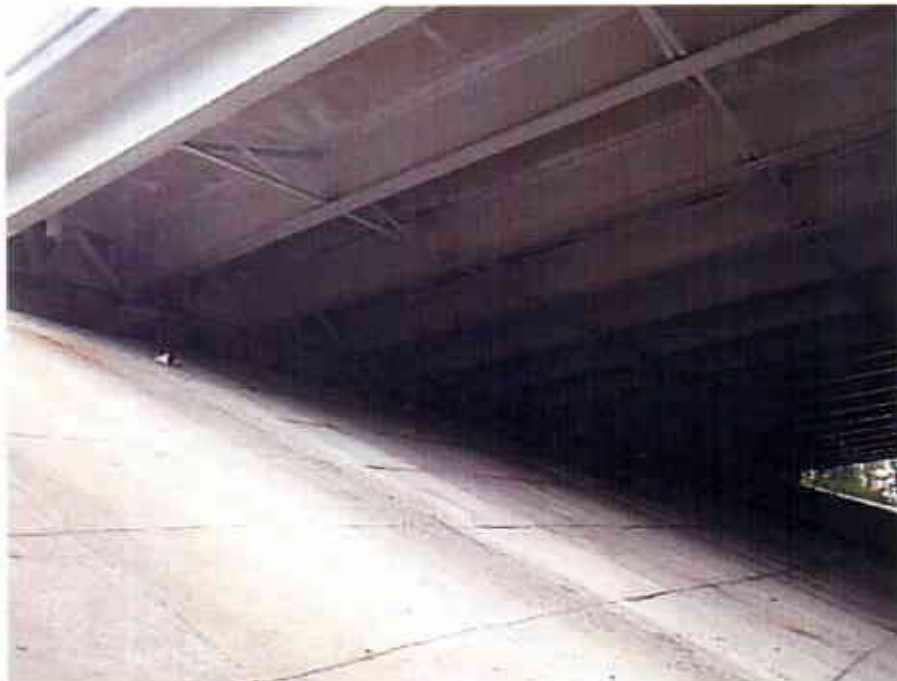
Photograph 44 View Looking North at the Underside of the East and West Bound Lanes of the Interstate 90 Bridge over Starkweather Avenue (CUY-90-1490L)
