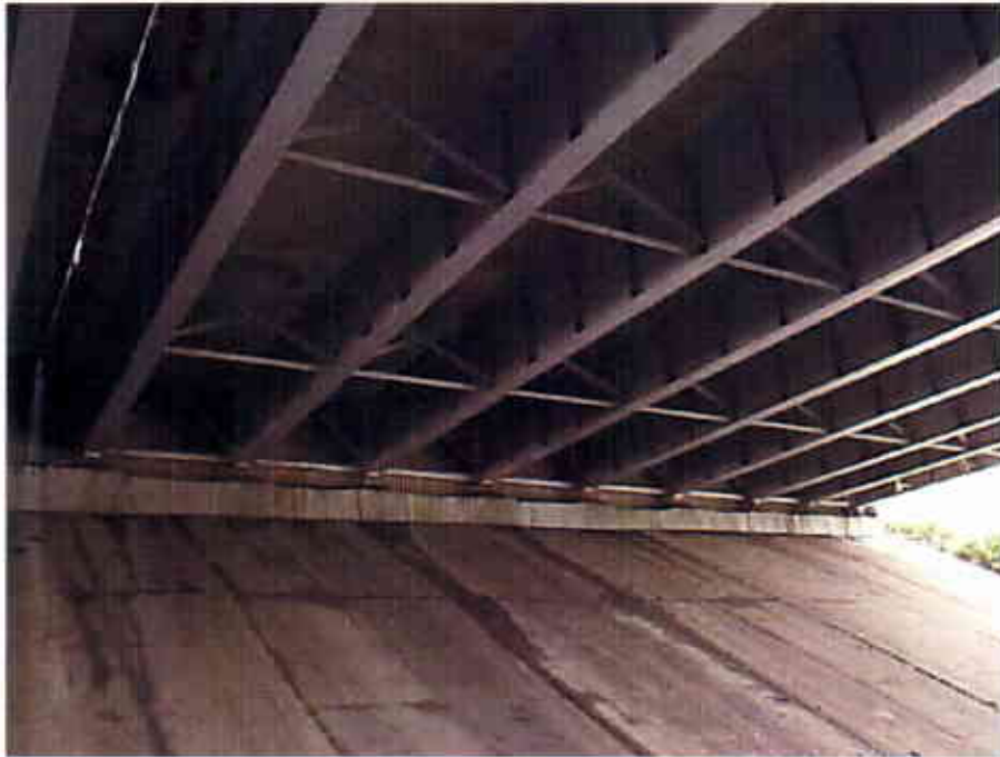
Photograph 06 View Looking East at the Underside of the East Bound Lanes of the Interstate 90 Bridge over East 14 th Street (CUY-90-1651R)
