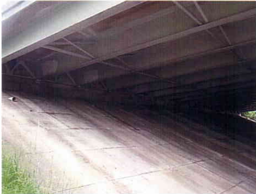
Photograph 47 View Looking South at the Underside of the East and West Bound Lanes of the Interstate 90 Bridge over Starkweather Avenue (CUY-90-1490R)
