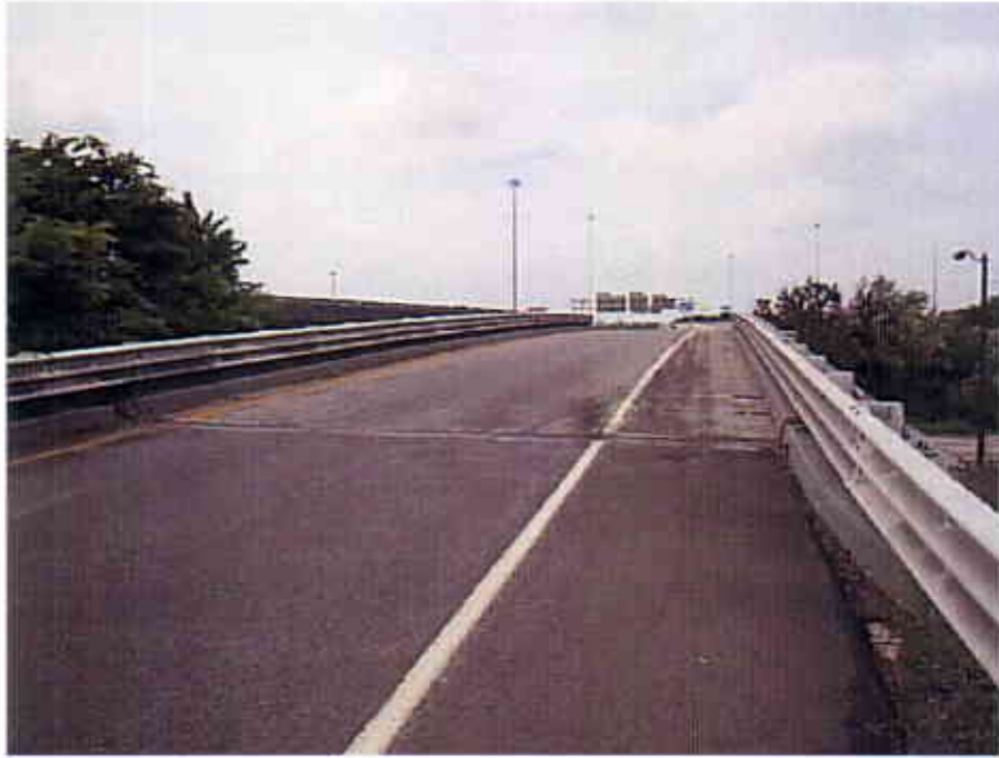
Photograph 15 View Looking West at the Top of the West Bound On Ramp of the Interstate 90 Bridge over East 9 th Street (CUY-90-1628EW)
