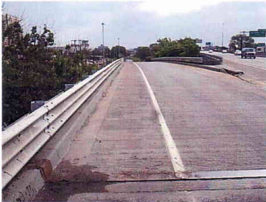
Photograph 16 View Looking East at the Top of the West Bound On Ramp of the Interstate 90 Bridge over East 9 th Street (CUY-90-1628EW)
