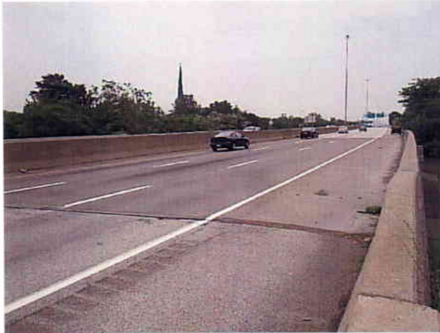
Photograph 43 View Looking South at the Top of the West Bound Lanes of the Interstate 90 Bridge over Starkweather Avenue (CUY-90-1490L)
