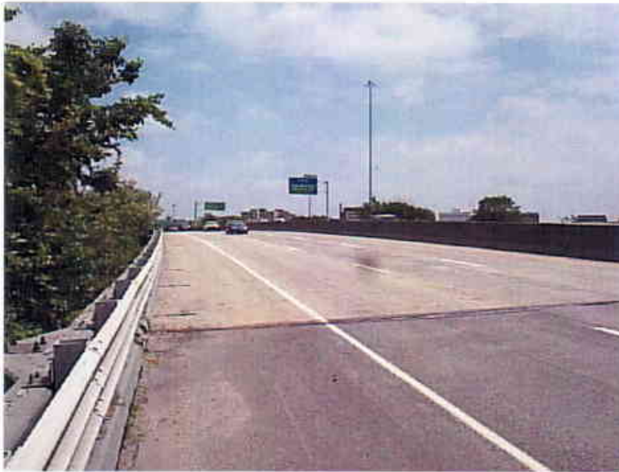
Photograph 13 View Looking East at the Top of the West Bound Lanes of the Interstate 90 Bridge over Ramps E-10 and E-8 (CUY-90-1640)
