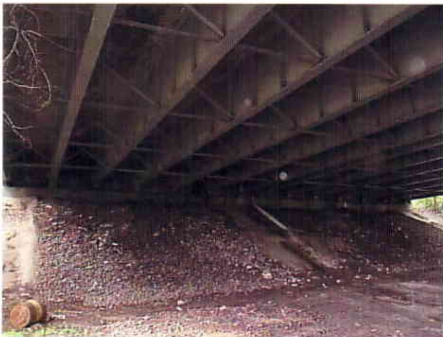
Photograph 14 View Looking West at the Underside of the East and West Bound Lanes of the Interstate 90 Bridge over Ramps E-10 and E-8 (CUY-90-1640)
