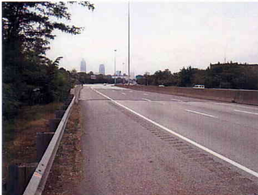
Photograph 42 View Looking North at the Top of the West Bound Lanes of the Interstate 90 Bridge over Starkweather Avenue (CUY-90-1490L)
