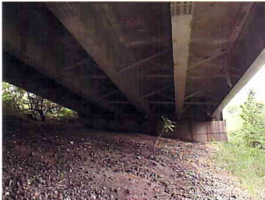
Photograph 50 View Looking West at the Underside of the East Bound Lanes of the Interstate 90 Bridge Ramp WN under I-71 Mainline Bridge (CUY-90-1463R)
