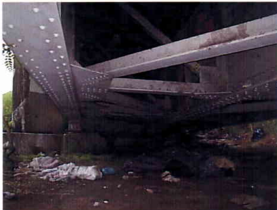
Photograph 30 View Looking West at the Underside of the East Bound Off Ramp Lane of the Interstate 90 Innerbelt Bridge over the Cuyahoga River (CUY-90-15.24)
