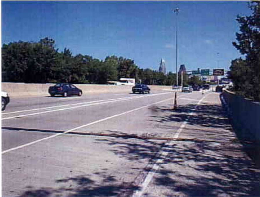
Photograph 41 View Looking North at the Top of the East Bound Lanes of the Interstate 90 Bridge over Kenilworth Avenue (CUY-90-1506)
