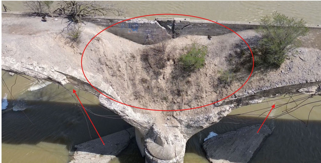
Typical condition of failed arch spandrels over piers. There are outer sections of the arch that have failed with only the rebar hanging. This condition below would justify a General Appraisal rating of a "0" if it occurred at a singular location. This issue is occurring at 50% of the pier locations.
