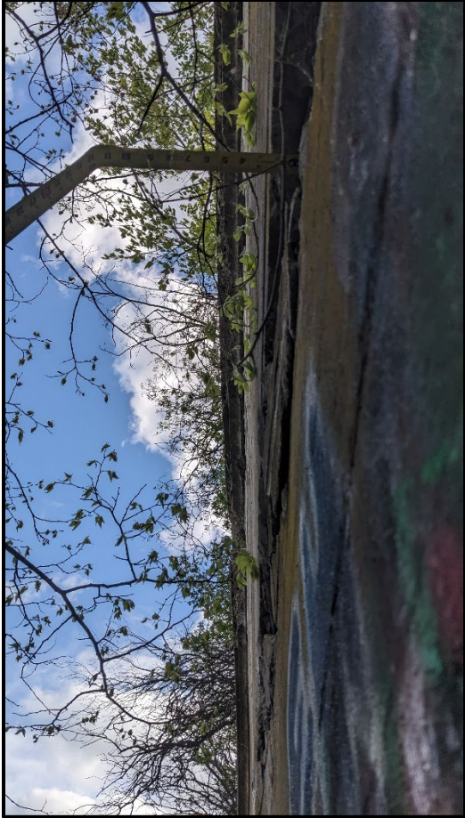
Photo 4 – East Spandrel Wall Movement 1.5 inches above Longitudinal Crack, Span 12.
