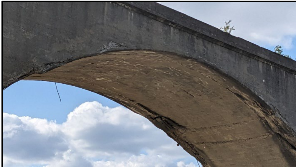
Photo 8 – Longitudinal Cracking with Calcium Hydroxide Efflorescence and Construction Joint Infiltration, Span 3.
