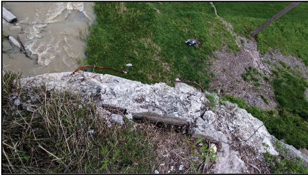
Photo 2 – Sparse Spandrel Wall Reinforcement, Span 2 East Spandrel Wall/
