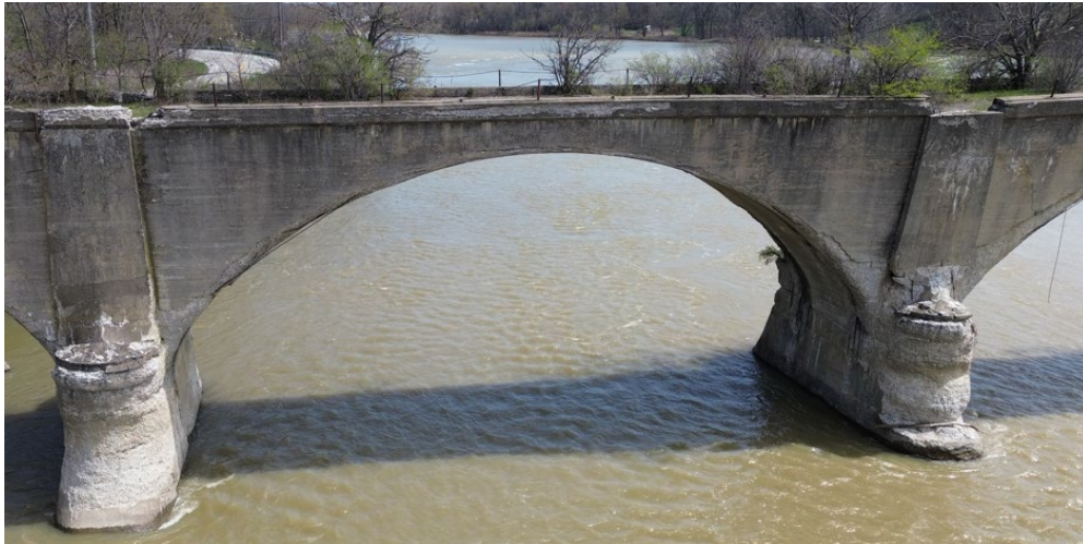
Span 11 (looking downstream) showing mostly sound spandrel walls. There is evidence that spandrel failure is starting to occur over the pier to the right.
