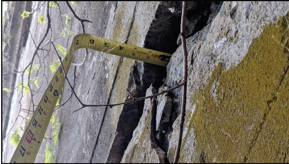
Photo 5 – Close-Up of East Spandrel Wall Movement 1.5 inches above Longitudinal Crack, Span 12.
