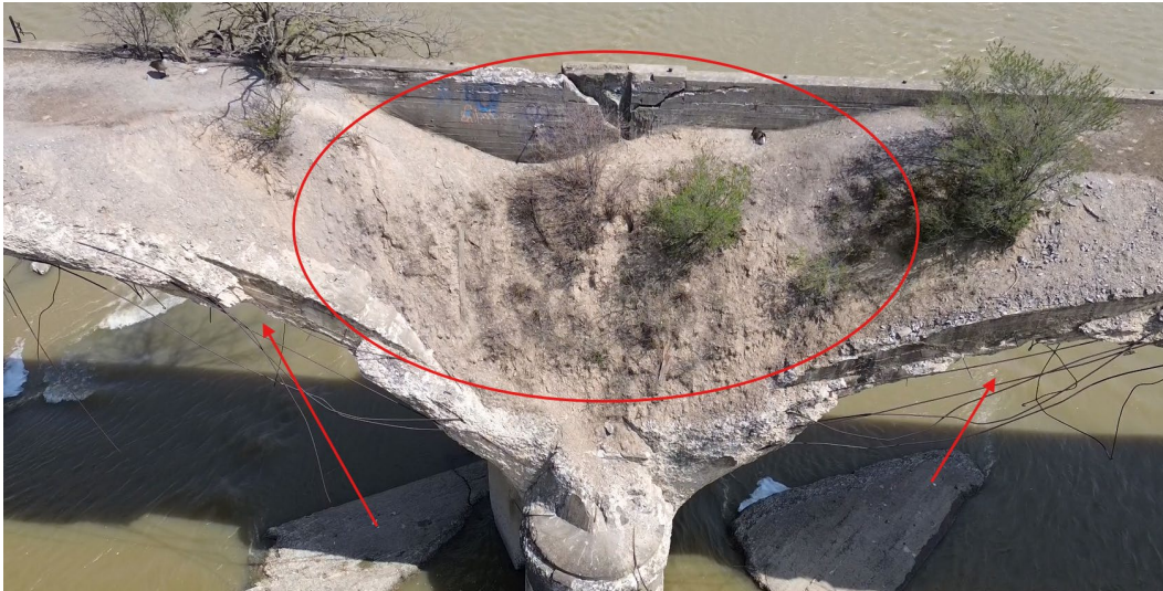
Typical condition of failed arch spandrels over piers. There are outer sections of the arch that have failed with only the rebar hanging. This condition below would justify a General Appraisal rating of a "0" if it occurred at a singular location. This issue is occurring at 50% of the pier locations.
