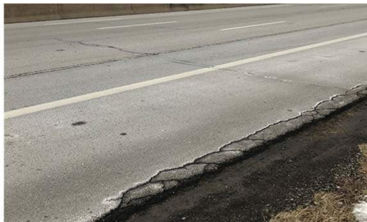
Photograph 1: IR-76 and IR-277 Pavement Wear
