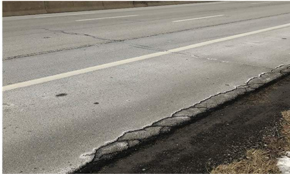
Photograph 1: IR-76 Pavement Wear
