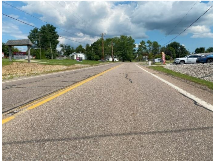
Picture 1: Looking SB on North Sandusky Street (SR 13) toward intersection with Upper Fredericktown Road / Crestview Avenue
